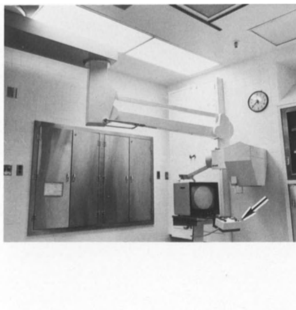
Fig. 4.6b. Overhead tube crane in parking position. No floor space is occupied. It can be moved in position much faster and more accurately than a portable machine. Remote control box with TV monitor on wheels (arrow). Tube output: 150 kV; focal spots: 0.6–1.2 mm with built-in automatic collimating system. Because of the larger energy output, shorter exposure times are required only (1/10–1/30th of a second).
