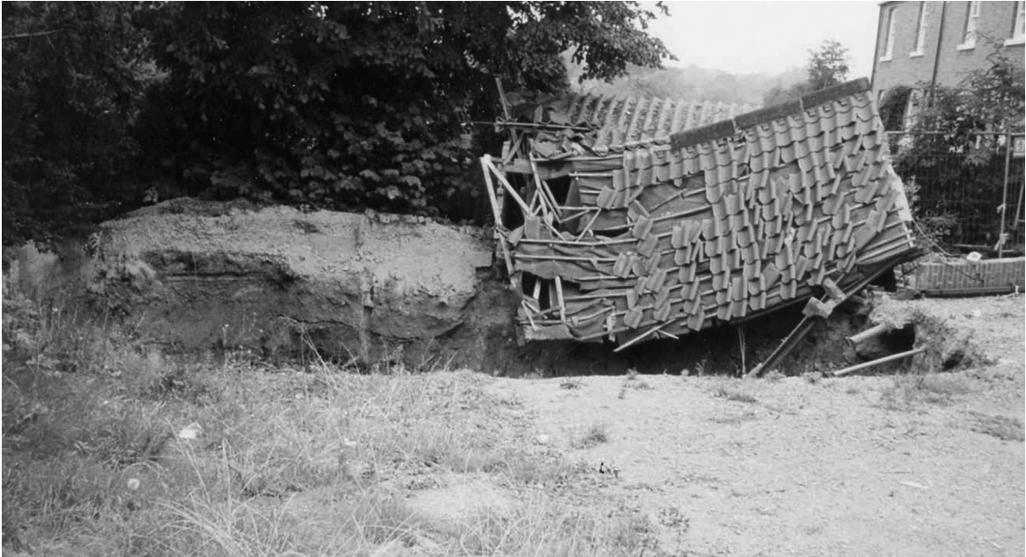
Fig. 8.1 A collapse doline formed in 1997 by failure of the roof of a flooded, natural cave in a bed of gypsum. The collapsed building was a double garage, adjoining a recently constructed detached house on Ure Bank Terrace, Ripon (North Yorkshire, UK). The gypsum bed containing the cave lies within a sequence of dolostone aquifers of Permian age, which are in turn overlain by a major sandstone aquifer of Permian age and permeable river gravels in hydraulic continuity with the River Ure. Vigorous cross-stratal groundwater flow is the root-cause of this dramatic subsidence feature. (Photograph courtesy of Dr John Lamont-Black.)
