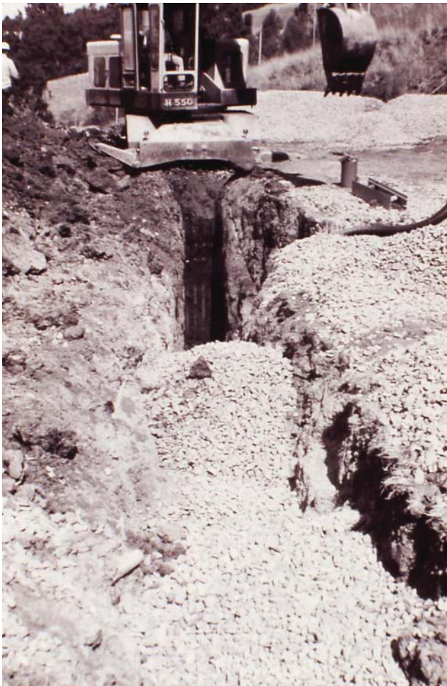
Figure 16.7 Trench drain at Lawrence Berkeley Laboratory.
