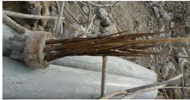
Figure 2.5 Rusted anchor strands in No. 3 Freeway landslide (Lee et al., 2012; photograph courtesy Taiwan Geotechnical Society and Ministry of Transportation, Taiwan).
