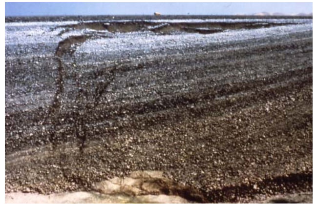
Figure 2.8 San Luis Dam upstream slope failure (U.S. government, Bureau of Reclamation photograph).
