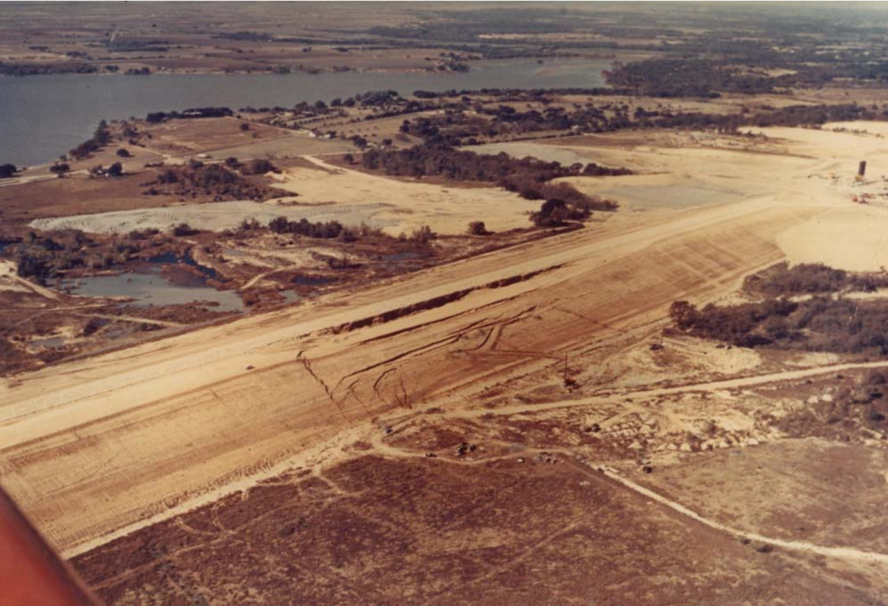
Figure 1.1 Slide in the downstream slope of the Waco Dam embankment (U.S. government, Corps of Engineers photograph).
