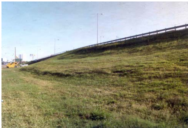
Figure 2.7 Slide in highway embankment near Houston, Texas. Embankment constructed of highly plastic clay.
