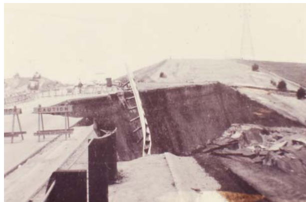
Figure 2.6 Interstate 80 embankment slope failure.
