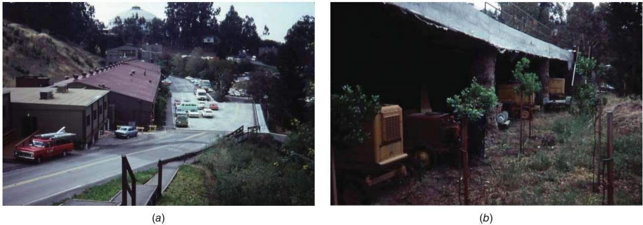
Figure 16.19 Landslide bridge at Lawrence Berkeley Laboratory, California: (a) top of bridge and (b) excavated area beneath bridge.
