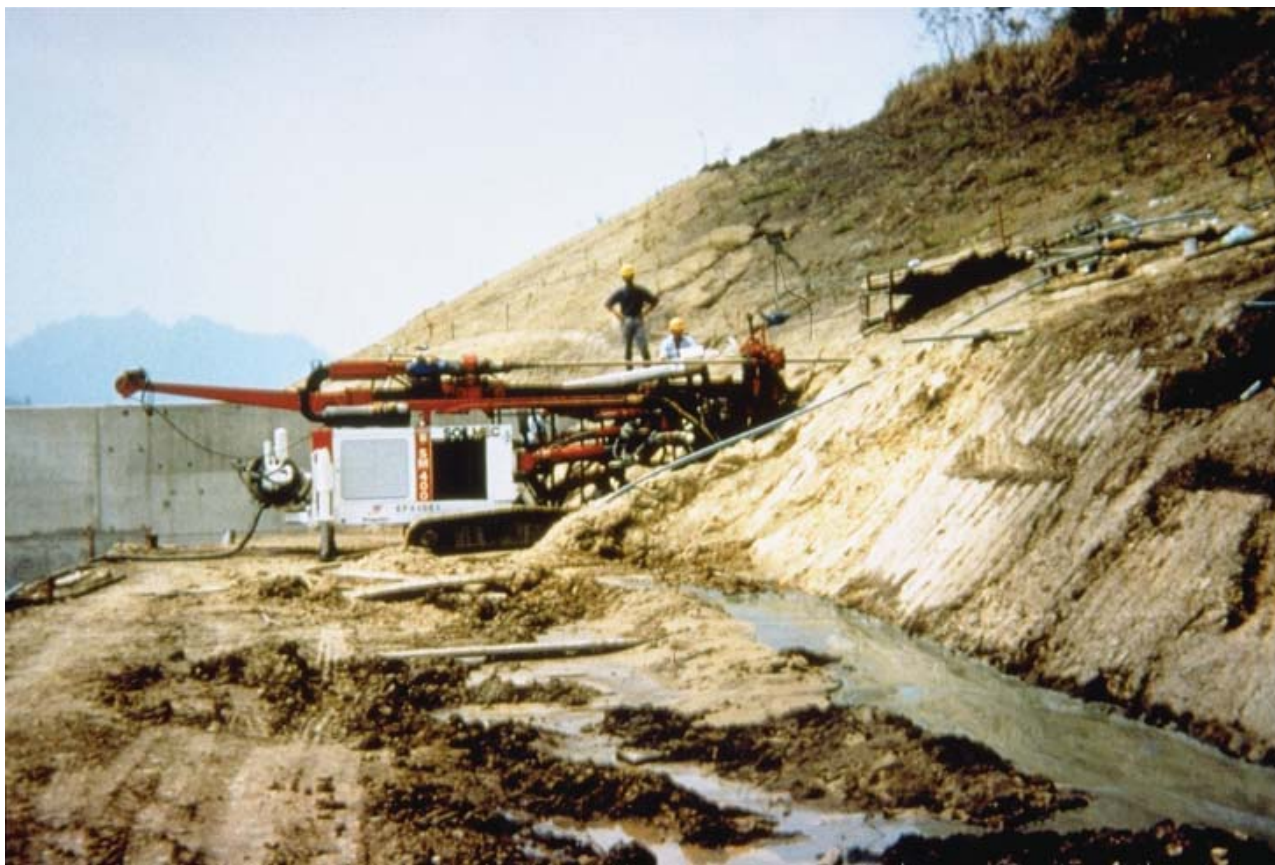
Figure 16.2 Drilling horizontal drains in the right abutment of La Esperanza Dam in Ecuador.
