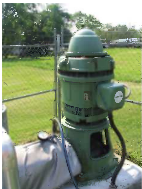
(a) Public water supply well with electrically powered line shaft turbine pump, USA [Photo: USGS].
