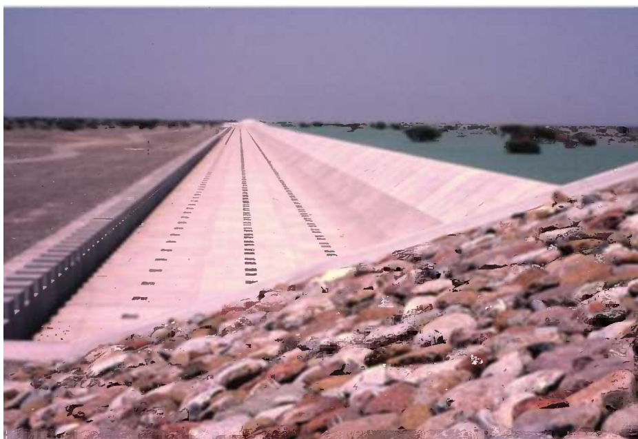
(b) Large recharge dam in the Batinah Plain, Oman [Photo: Jac van der Gun]. Flood water is retained by the dam and is subsequently released in a controlled way to recharge the aquifer zone downstream.
