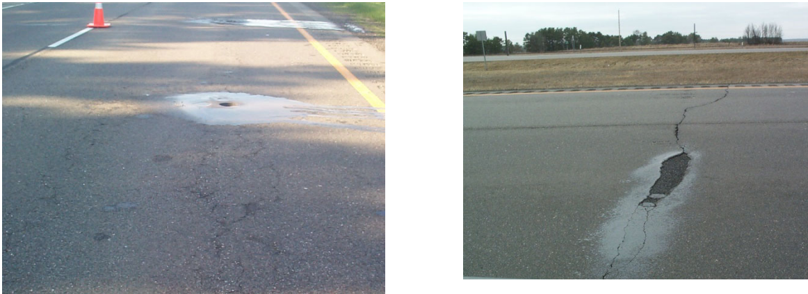
Figure 1. T.H. 10 - 5% RAS: May 2008 (Left) and March 2007 (Right) (1)
