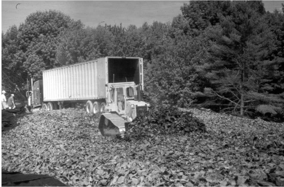
Fig. 2 Catipillar D-4 spreading tire shreds for lightweight embankment fill at Portland Jetport Interchange
