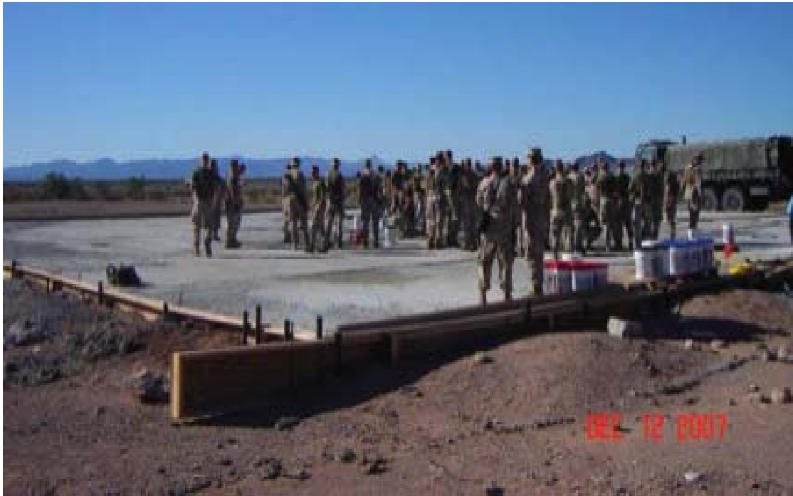
Figure 8. Marine Corps Engineers training for fast track construction and repair prior to deployment. Marine Corps Base Concrete Installation
