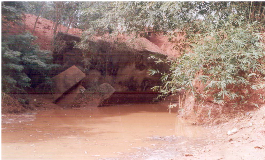
Figure 1: Eroded Roadside Retaining Wall and Roadside Embankment at Amatutu, Anambra State
