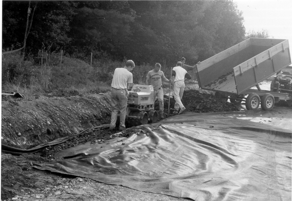
Fig. 8 Placing and compacting tire shreds in edge drain for Witter Farm Road.
