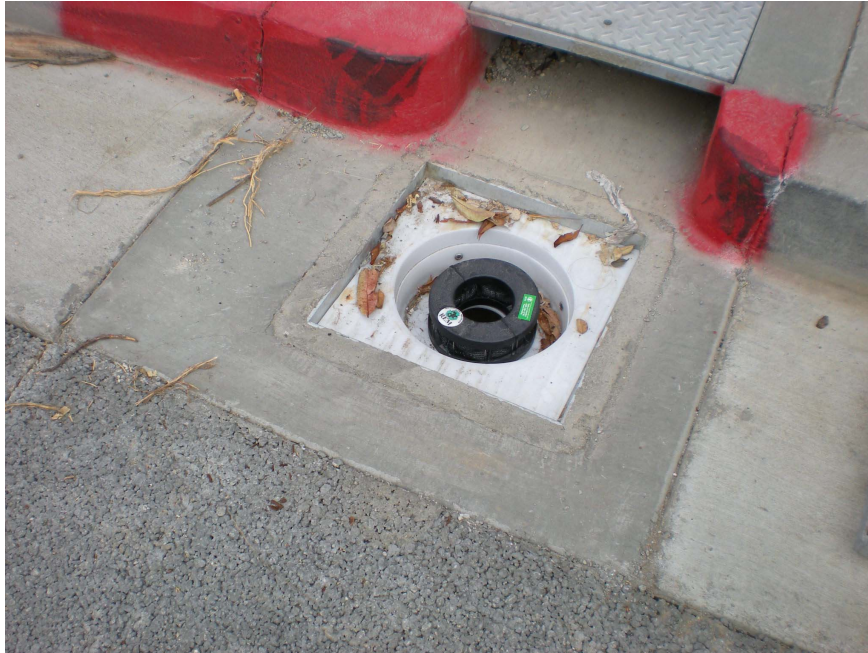
Figure 4. Gutter catch basin with filter to pre-treat/screen runoff as it flows into the basin and then into the sub-surface storage chamber.
