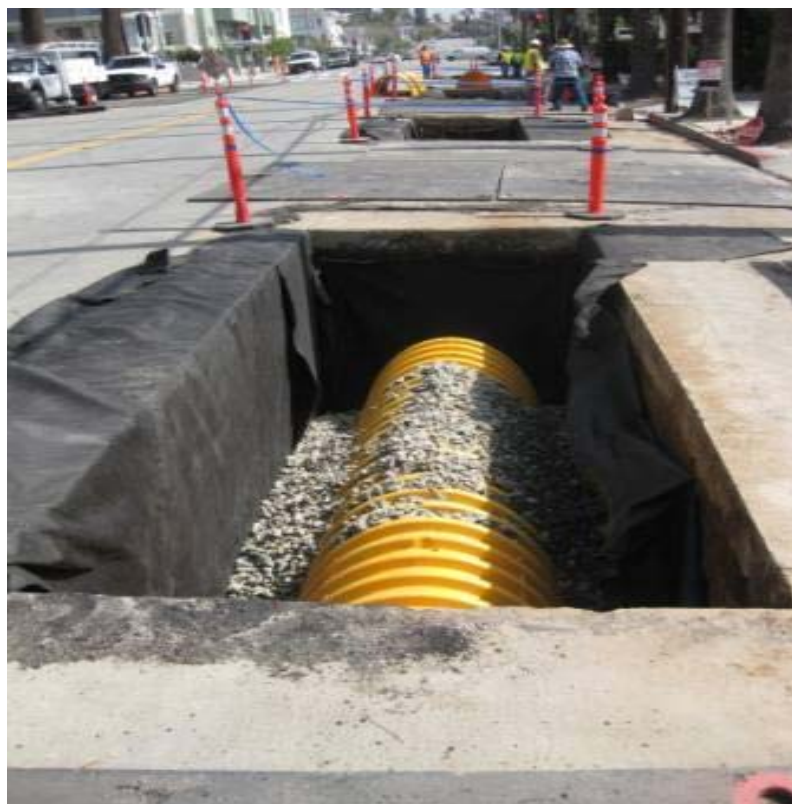
Figure 5. Sub-surface storage chamber under parking lane.
