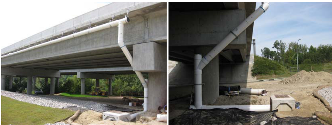
Figure 3. Pictures of water delivery systems for bioretention and bioswale.
