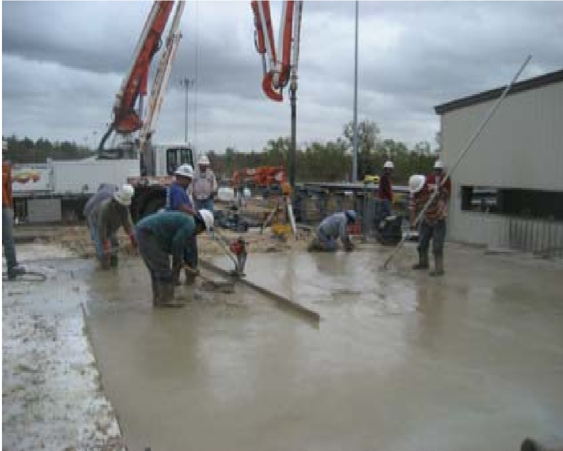
Figure 5. Construction of base for a heat treating facility in Houston, Texas. Cycling of temperatures caused severe breakdown of conventional concrete.
