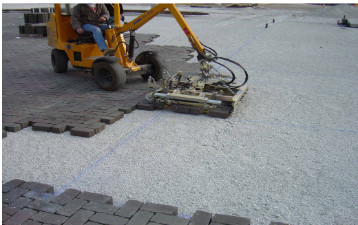
Figure 7. Mechanized PICP installation is increasingly used to decrease time and installation costs compared to manual installation.
