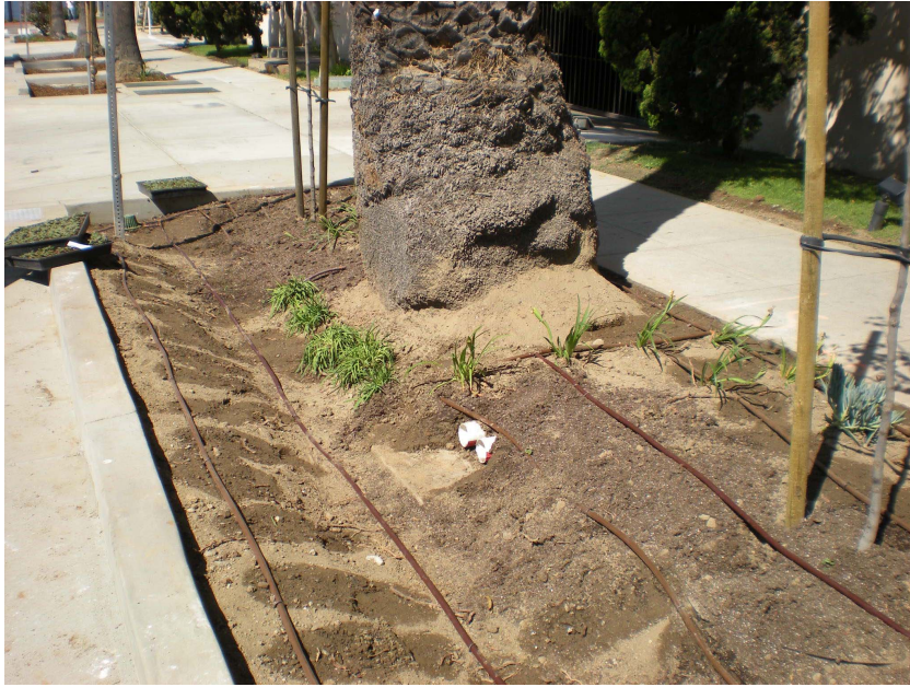
Figure 6. Depressed parkways receive runoff from gutter through curb cuts or roof downspout pipes (note 2 white pipes in center of parkway from adjacent building roof).
