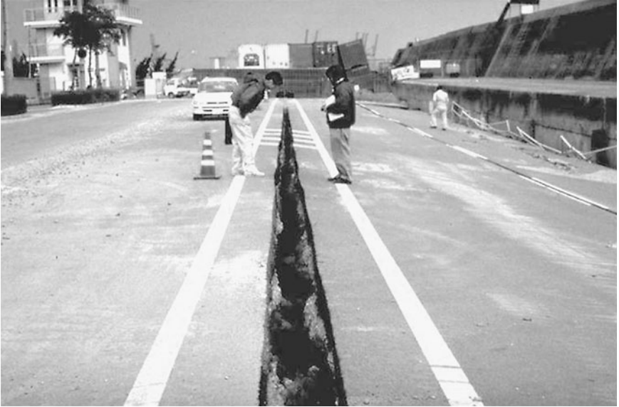
FIGURE 3.33 Damage on Port Island caused by retaining wall movement during the Kobe earthquake on January 17, 1995. (Photograph from the Kobe Geotechnical Collection, EERC, University of California, Berkeley.)
