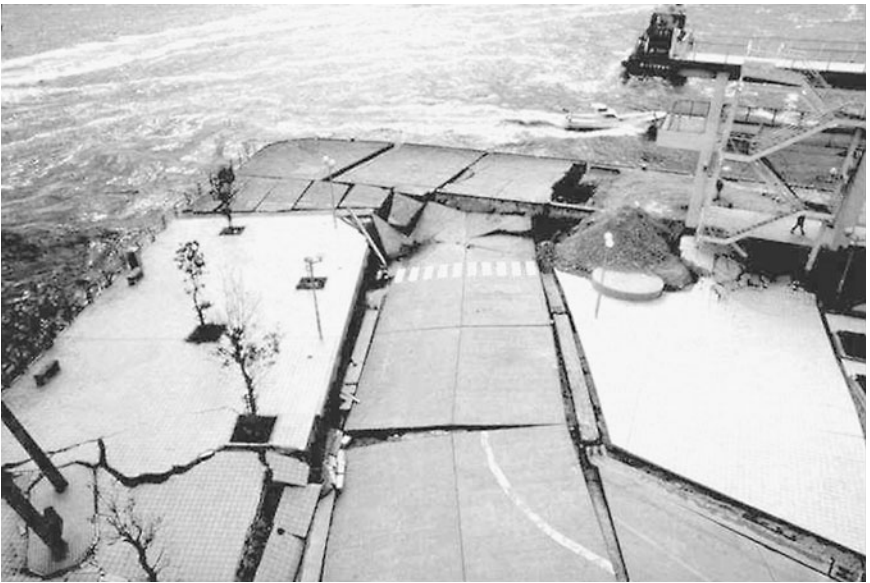
FIGURE 3.29 Settlement and lateral spreading damage due to retaining wall movement caused by the Kobe earthquake on January 17, 1995. The location is near the northwest corner of the Port Island Bridge. (Photograph from the Great Hanshin Bridge Collection, EERC, University of California, Berkeley.)
