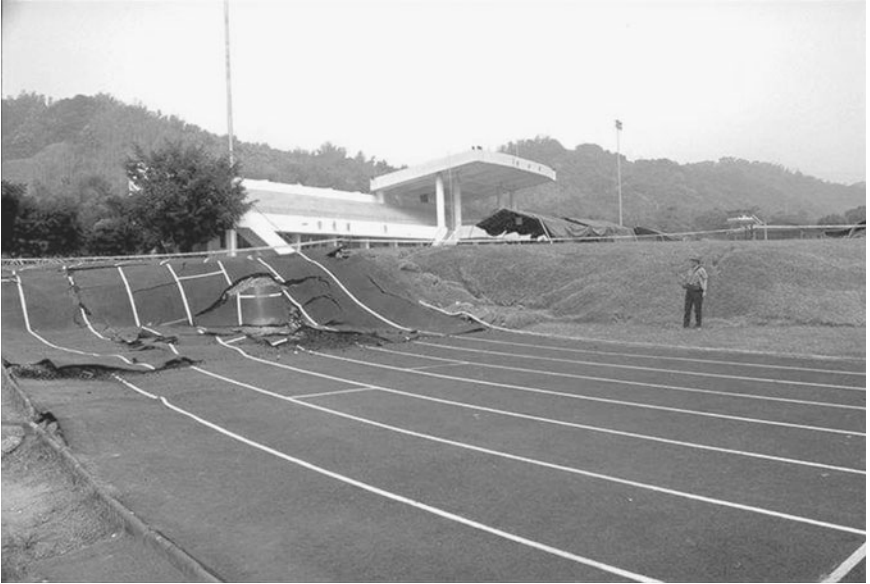
FIGURE 3.5 Overview of damage to the Kuang Fu Elementary School by surface fault rupture associated with the Chi-chi (Taiwan) earthquake on September 21, 1999. (Photograph from the Taiwan Collection, EERC, University of California, Berkeley.)
