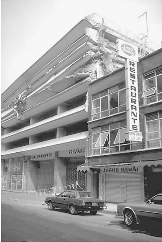
FIGURE 4.17 Pancaking of the upper floors of a parking garage during the Michoacan earthquake in Mexico on September 19, 1985. Note that the restaurant building provided additional lateral support which enabled the lower three floors of the parking garage to resist the collapse. (Photograph from the Steinbrugge Collection, EERC, University of California, Berkeley.)
