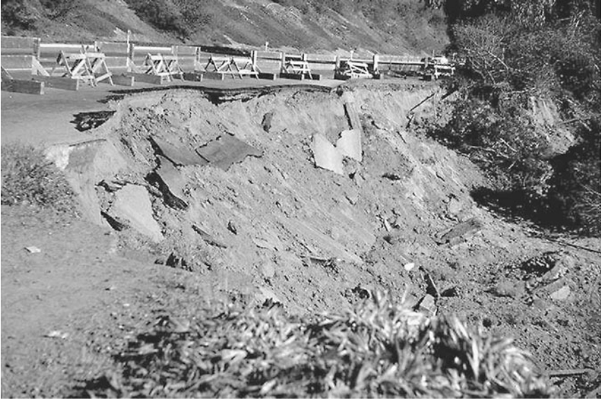
FIGURE 9.35 One of several earthquake-induced slides along Skyline Boulevard at Lake Merced, San Francisco. The slides were caused by the Daly City earthquake in California on March 22, 1957. (Photograph from the Steinbrugge Collection, EERC, University of California, Berkeley.)
