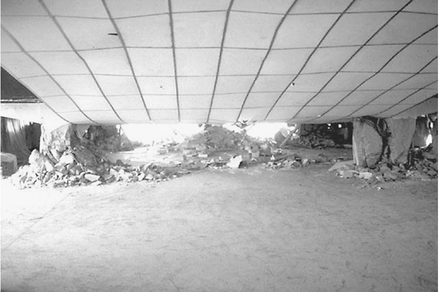
FIGURE 4.3 Torsional failure of the second story of the Hotel Terminal. The torsional failure occurred during the Gualan earthquake in Guatemala on February 4, 1976. (Photograph from the Godden Collection, EERC, University of California, Berkeley.)
