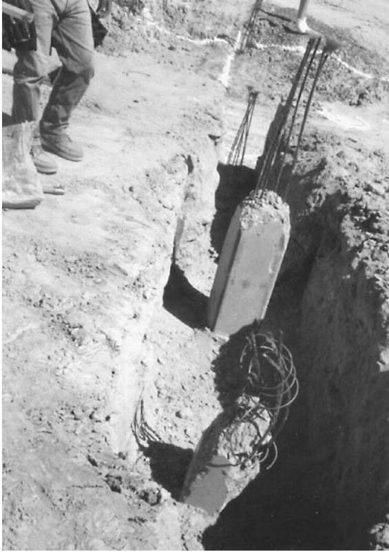
FIGURE 13.30 The prestressed concrete pile at the bottom of the picture is the same pile shown in Fig. 13.23. The pile near the center of the photograph is the replacement pile. The broken pile and the replacement pile will be attached to the grade beam.
