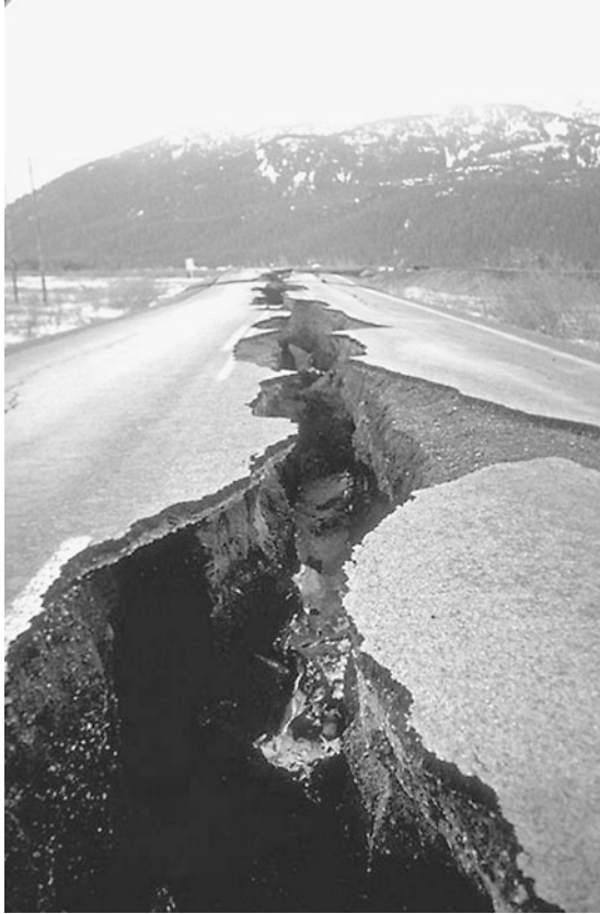
FIGURE 3.54 Cracking of the Anchorage–Portage highway. The small highway embankment experienced lateral movement during the Prince William Sound earthquake in Alaska on March 27, 1964. (Photograph from the Steinbrugge Collection, EERC, University of California, Berkeley.)
