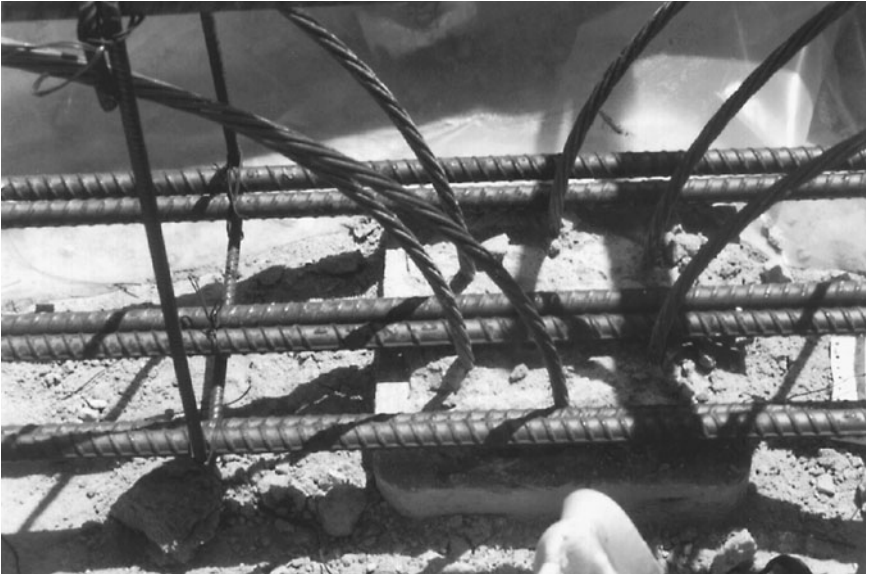
FIGURE 13.33 Close-up view of the top of a prestressed pile with the steel reinforcement from the grade beam positioned on top of the pile. The strands from the pile are attached to the steel reinforcement in the grade beam.
