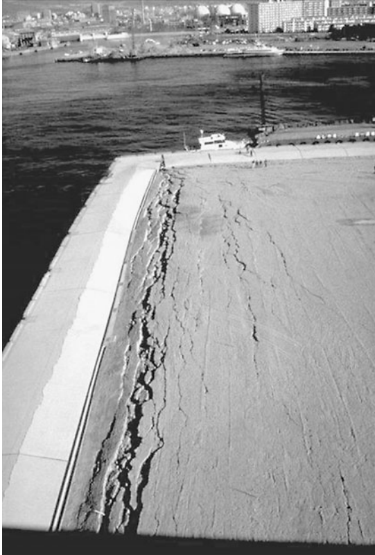
FIGURE 3.36 The liquefaction-induced retaining wall movement was caused by the Kobe Earthquake on January 17, 1995. Both lateral spreading fissures and sporadic sand boils were observed behind the retaining wall. The site is near the pier of Nishihomiya Bridge, which previously supported the collapsed expressway section. (Photograph from the Kobe Geotechnical Collection, EERC, University of California, Berkeley.)
