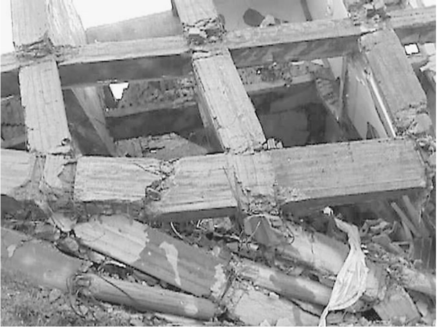
FIGURE 4.10 Building collapse caused by a soft story at the first-floor level. The damage occurred during the Izmit earthquake in Turkey on August 17, 1999. (Photograph by Mehmet Celebi, USGS.)
