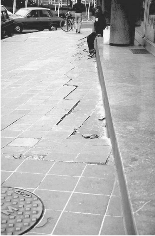
FIGURE 7.11 Settlement caused by the building rocking back and forth during the Michoacan earthquake in Mexico on September 19, 1985. (Photograph from the Steinbrugge Collection, EERC, University of California, Berkeley.)
