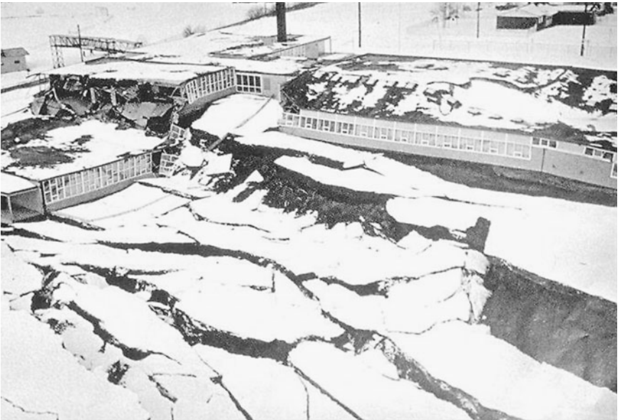
FIGURE 3.52 Overview of damage to the Government Hill School located at the head of a landslide caused by the Prince William Sound earthquake in Alaska on March 27, 1964. (Photograph from the Steinbrugge Collection, EERC, University of California, Berkeley.)
