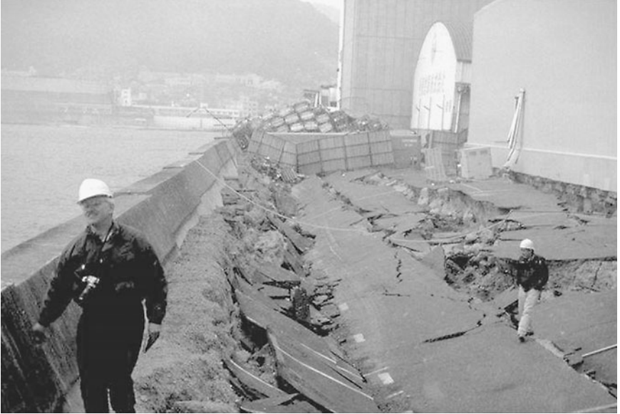
FIGURE 3.28 Lateral retaining wall movement due to liquefaction during the Kobe earthquake on January 17, 1995. As the retaining wall has moved outward, the ground surface has dropped. The site is adjacent to the east end of the Higashi Kobe Bridge. (Photograph from the Great Hanshin Bridge Collection, EERC, University of California, Berkeley.)
