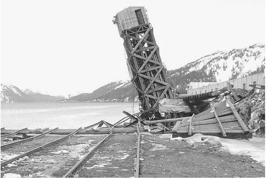
FIGURE 4.2 Close-up view of the tilted tower shown in Fig. 4.1. The tilting of the tower was caused by the washing away of soil due to a tsunami generated during the Prince William Sound earthquake in Alaska on March 27, 1964. (Photograph from the Steinbrugge Collection, EERC, University of California, Berkeley.)
