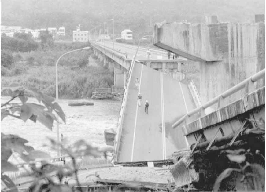
FIGURE 3.10 Another view of the collapsed bridge north of Fengyuen caused by surface fault rupture associated with the Chi-chi (Taiwan) earthquake on September 21, 1999. (Photograph from the USGS Earthquake Hazards Program, NEIC, Denver.)
