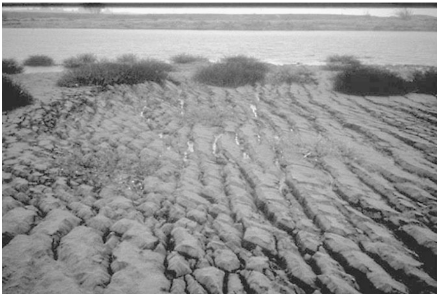
FIGURE 3.41 Lateral spreading caused by the Loma Prieta, California, earthquake on October 17, 1989. (Photograph from the Loma Prieta Collection, EERC, University of California, Berkeley.)
