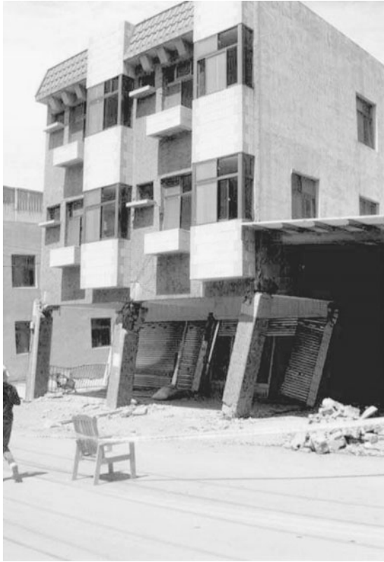
FIGURE 4.5 Damage due to a soft story at the ground floor. The damage occurred during the Chi-chi earthquake in Taiwan on September 21, 1999. (Photograph from the USGS Earthquake Hazards Program, NEIC, Denver.)
