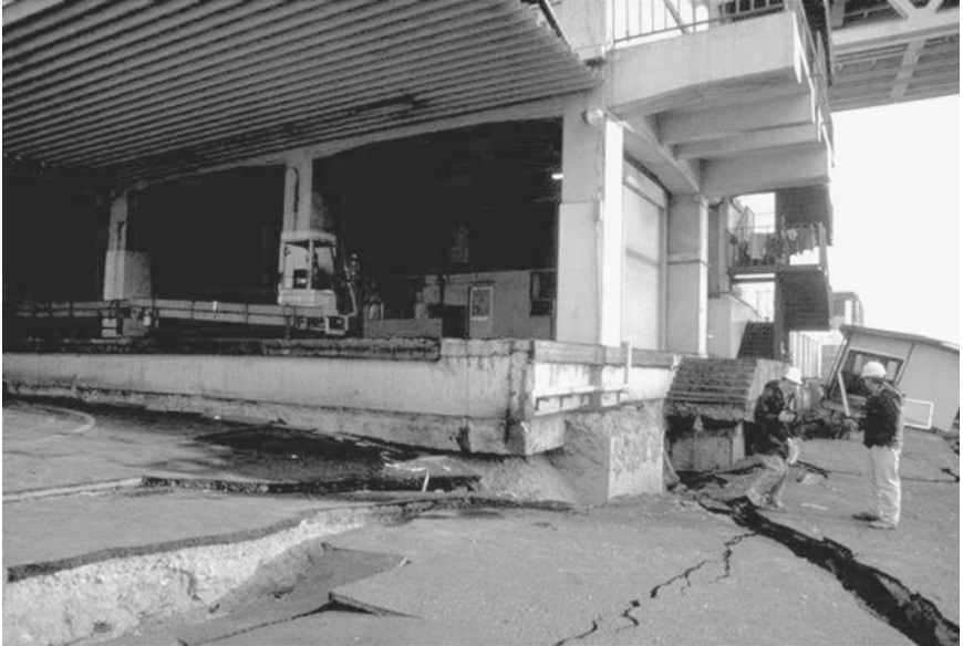
FIGURE 3.35 Settlement caused by lateral movement of a retaining wall during the Kobe earthquake on January 17, 1995. The industrial building is supported by a pile foundation. The Higashi Kobe cable-stayed bridge is visible in the upper right corner of the photograph. (Photograph from the Great Hanshin Bridge Collection, EERC, University of California, Berkeley.)
