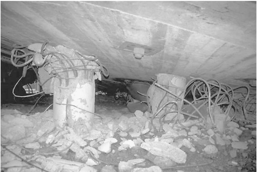
FIGURE 4.13 Close-up view of the columns that had supported the elevated gas storage tank shown in Fig. 4.12. The columns did not have adequate shear resistance and were unable to support the gas storage tank during the Izmit earthquake in Turkey on August 17, 1999. (Photograph from the Izmit Collection, EERC, University of California, Berkeley.)
