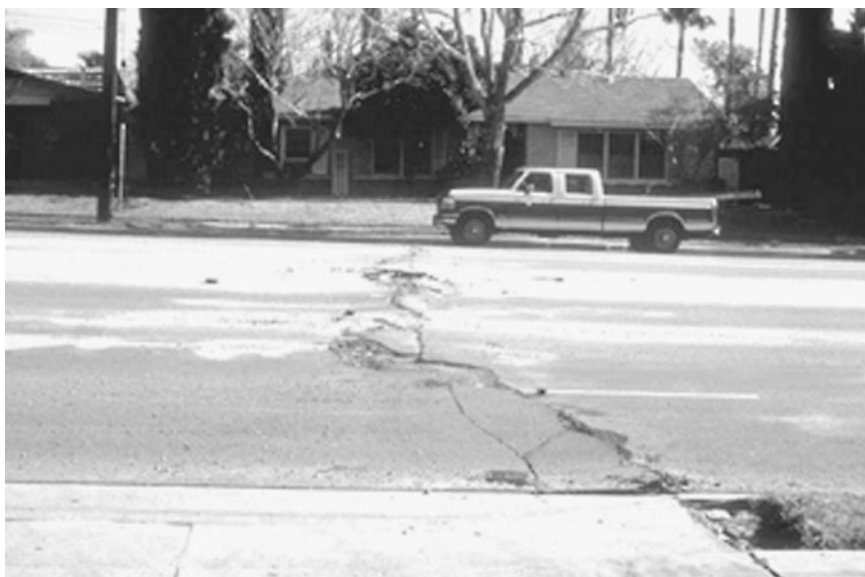
FIGURE 11.5 Localized compression feature and pavement damage caused by the Northridge earthquake, in California, on January 17, 1994. (Photograph from the Northridge Collection, EERC, University of California, Berkeley.)
