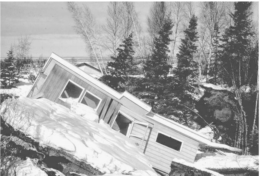
FIGURE 3.48 Damage caused by movement of the Turnagain Heights landslide during the Prince William Sound earthquake in Alaska on March 27, 1964. (Photograph from the Steinbrugge Collection, EERC, University of California, Berkeley.)
