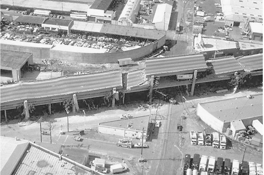
FIGURE 4.27 Overview of the collapse of the Cypress Street Viaduct caused by the Loma Prieta earthquake in California on October 17, 1989. (From USGS.)
