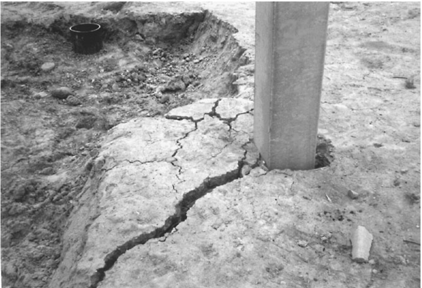
FIGURE 13.22 Lateral displacement of a prestressed concrete pile during the driving operations.
