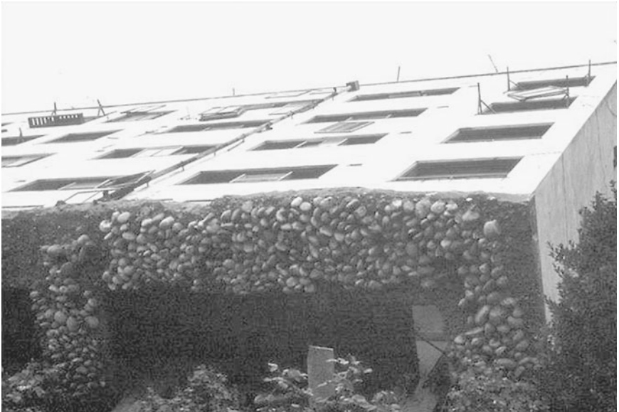
FIGURE 3.21 View of the bottom of a Kawagishi-cho apartment building located in Niigata, Japan. The building suffered a liquefaction-induced bearing capacity failure during the Niigata earthquake on June 16, 1964. (Photograph from the Steinbrugge Collection, EERC, University of California, Berkeley.)
