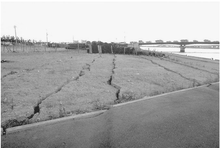
FIGURE 3.27 Ground cracks caused by lateral retaining wall movement due to liquefaction during the Kobe earthquake on January 17, 1995. The site is near Nishinomiya Port and consists of reclaimed land. (Photograph from the Great Hanshin Bridge Collection, EERC, University of California, Berkeley.)
