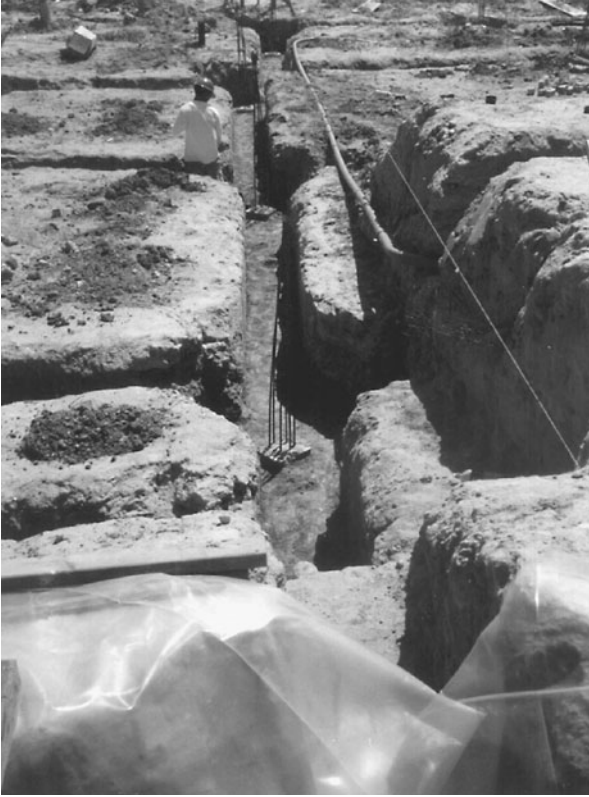
FIGURE 13.31 The excavation for the grade beams is complete, and the tops of the prestressed piles are trimmed so that they are relatively flush.
