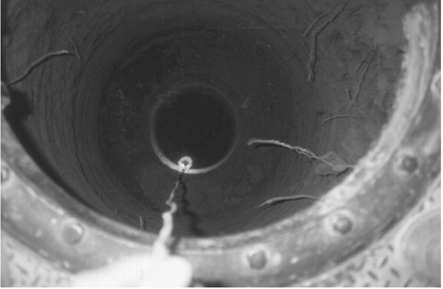
FIGURE 13.9 A light has been lowered to the bottom of the pier to observe embedment conditions.
