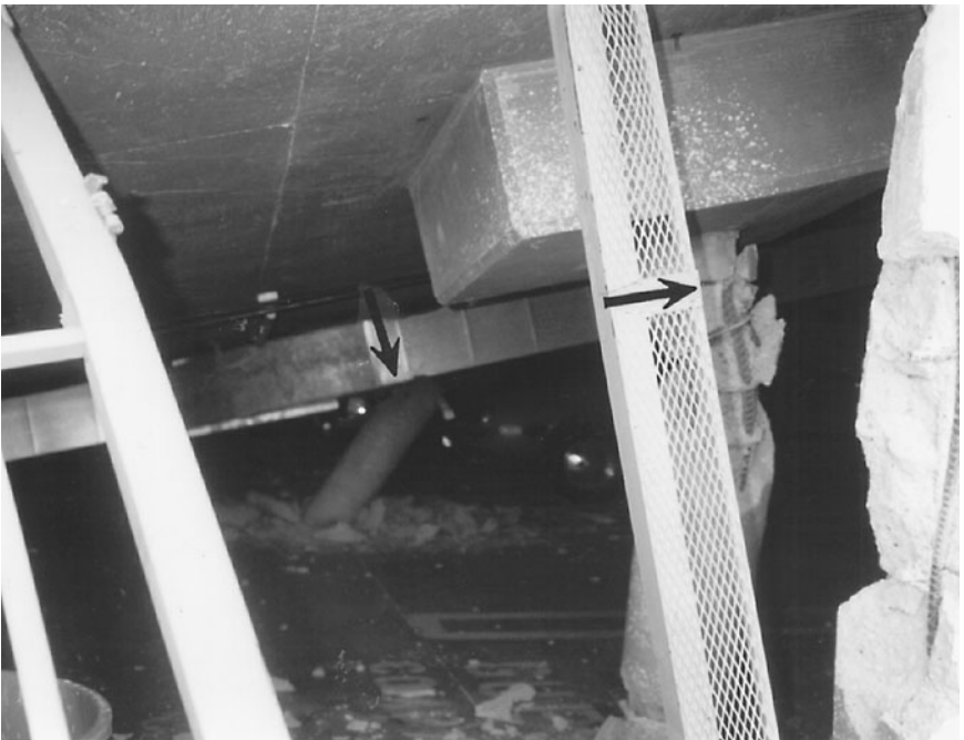
FIGURE 4.7 View inside the collapsed first-floor parking garage (the arrows point to the columns). The building collapse occurred during the Northridge earthquake in California on January 17, 1994.
