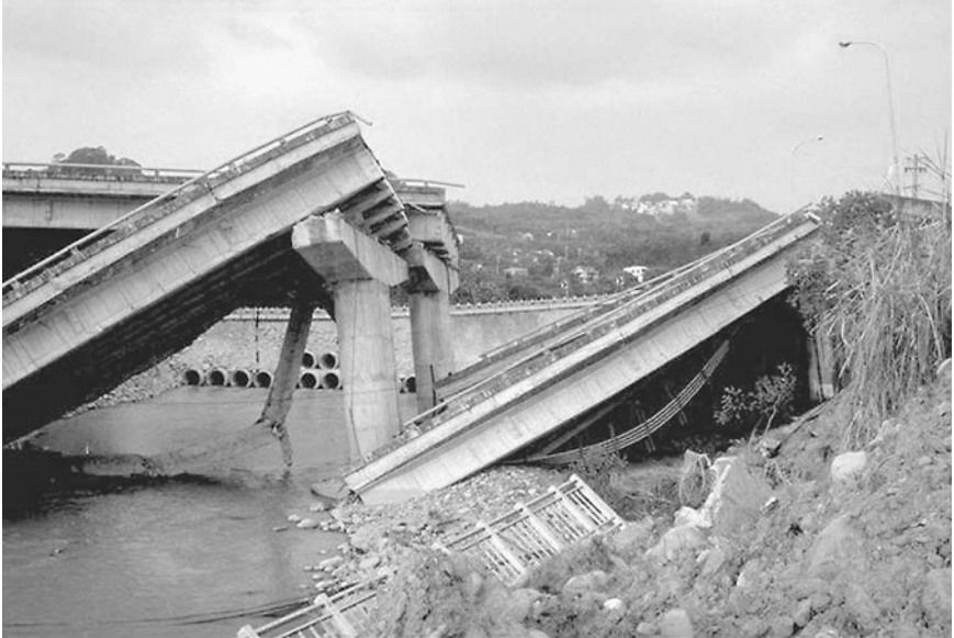
FIGURE 9.37 Earthquake-induced landslide movement that damaged the south abutment of the Shih-Wui Bridge. The landslide was caused by the Chi-chi (Taiwan) earthquake on September 21, 1999. (Photograph from the Taiwan Collection, EERC, University of California, Berkeley.)
