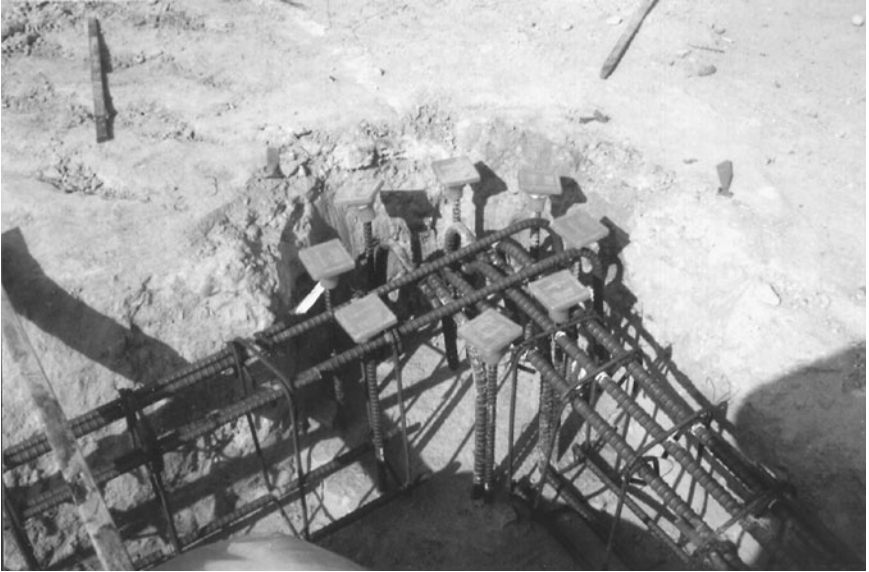
FIGURE 13.13 Corner of the building where the steel reinforcement from the two grade beams has been attached to the steel reinforcement from the pier.
