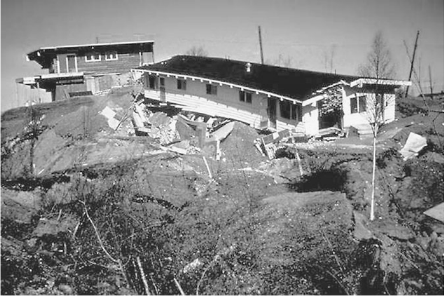
FIGURE 3.47 Damage caused by movement of the Turnagain Heights landslide during the Prince William Sound earthquake in Alaska on March 27, 1964. (Photograph from the Godden Collection, EERC, University of California, Berkeley.)
