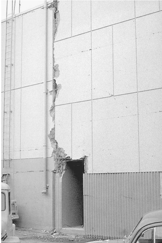
FIGURE 4.20 Pounding damage to the Anchorage-Westward Hotel caused by the Prince William Sound earthquake in Alaska on March 27, 1964. The building on the right half of the photograph is the 14-story hotel, while the building visible on the left half of the photograph is the ballroom. (Photograph from the Steinbrugge Collection, EERC, University of California, Berkeley.)
