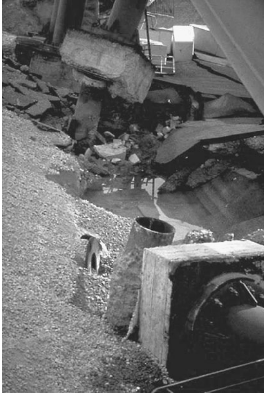
FIGURE 13.35 The top of the steel pile separated from the concrete pile cap during the Kobe earthquake on January 17, 1995. (Photograph from the Kobe Geotechnical Collection, EERC, University of California, Berkeley.)
