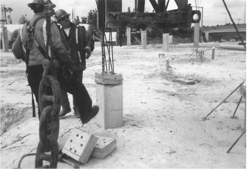
FIGURE 13.21 A prestressed concrete pile has been successfully driven to the bearing strata. The wood block shown on top of the concrete pile was used as a cushion to protect the pile top from being crushed during the driving operation.
