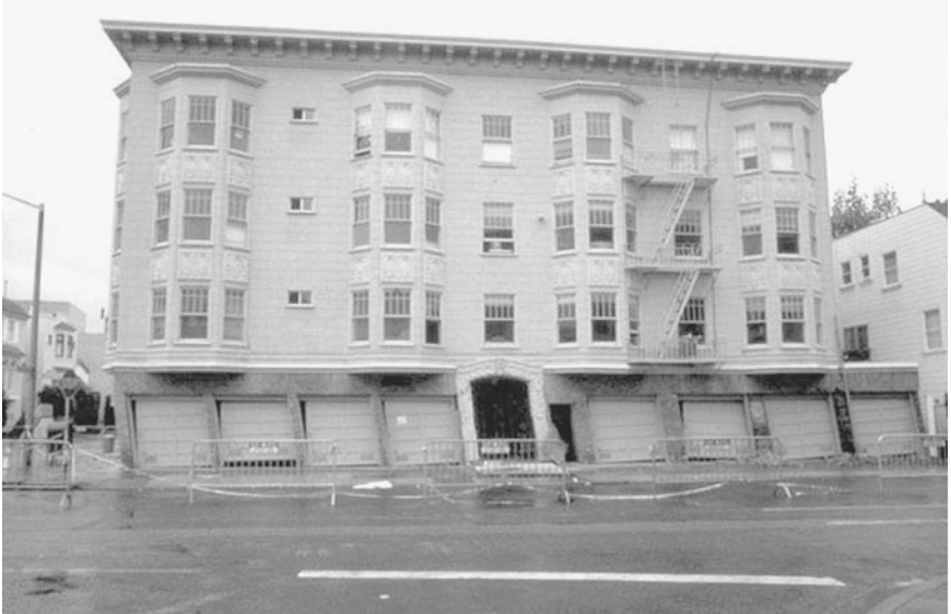
FIGURE 4.8 Damage caused by a soft story due to a parking garage on the first floor. The damage occurred during the Loma Prieta earthquake in California on October 17, 1989. (Photograph from the Loma Prieta Collection, EERC, University of California, Berkeley.)
