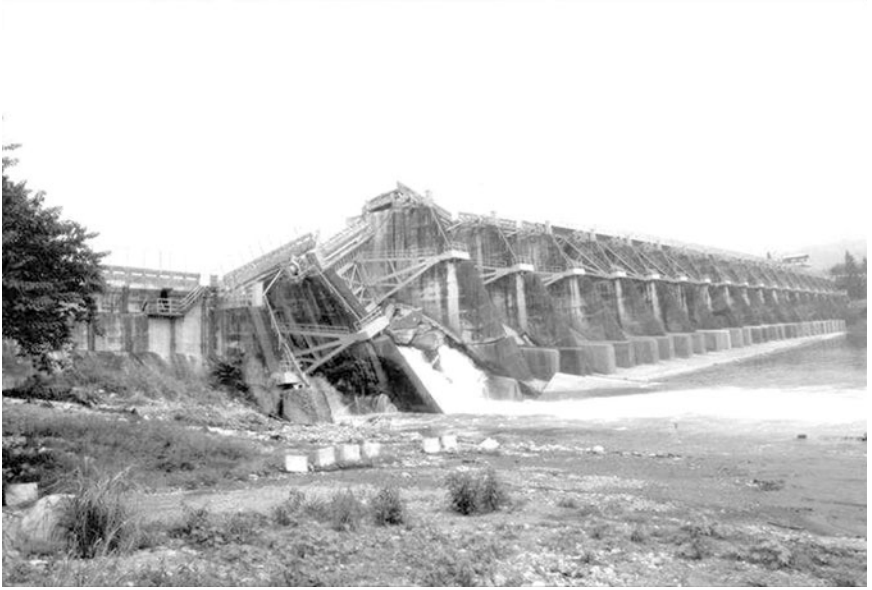
FIGURE 3.3 Overview of a dam damaged by surface fault rupture associated with the Chi-chi (Taiwan) earthquake on September 21, 1999. (Photograph from the Taiwan Collection, EERC, University of California, Berkeley.)
