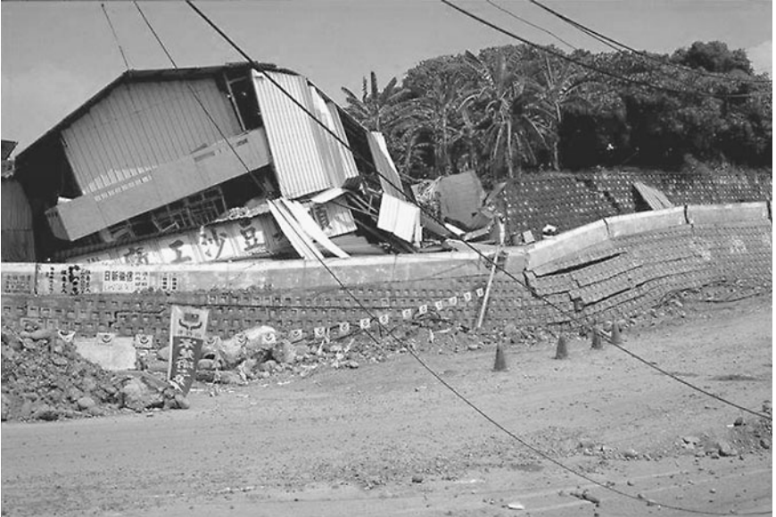
FIGURE 3.8 Retaining wall located north of Chung-Hsing (Jung Shing). At this site, the surface fault rupture associated with the Chi-chi (Taiwan) earthquake on September 21, 1999, has caused both vertical and horizontal displacement of the retaining wall. (Photograph from the Taiwan Collection, EERC, University of California, Berkeley.)
