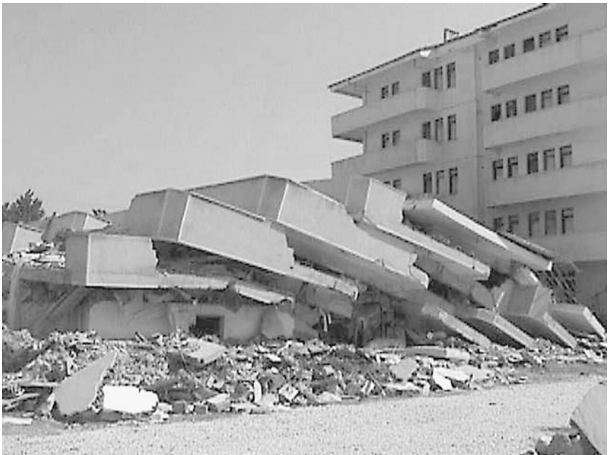
FIGURE 4.14 Pancaking of a building during the Izmit earthquake in Turkey on August 17, 1999. (Photograph by Mehmet Celebi, USGS.)
