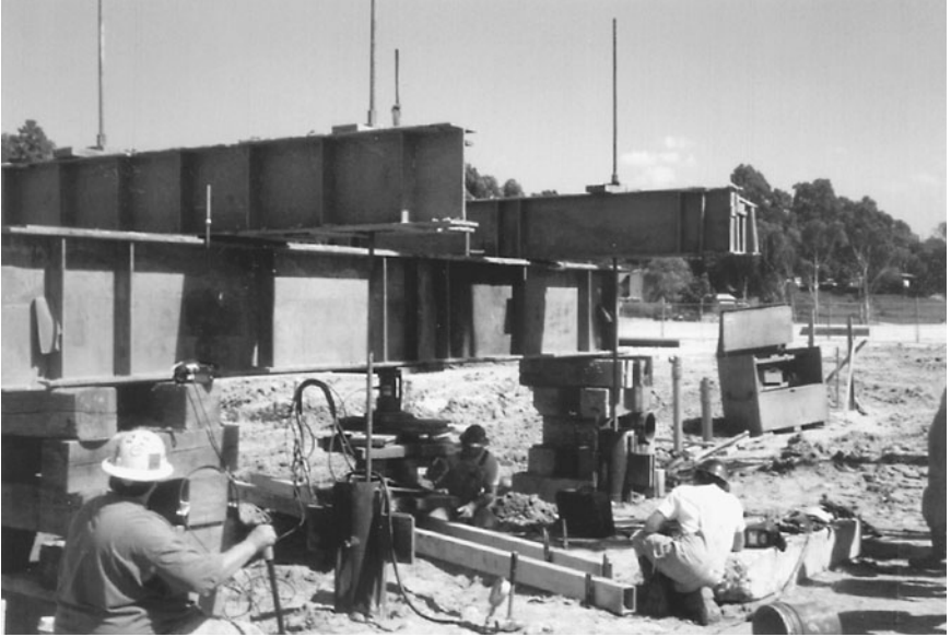
FIGURE 13.26 Pile load tests. The reaction frame has been set up, and the hydraulic jack and load cell are in place.
