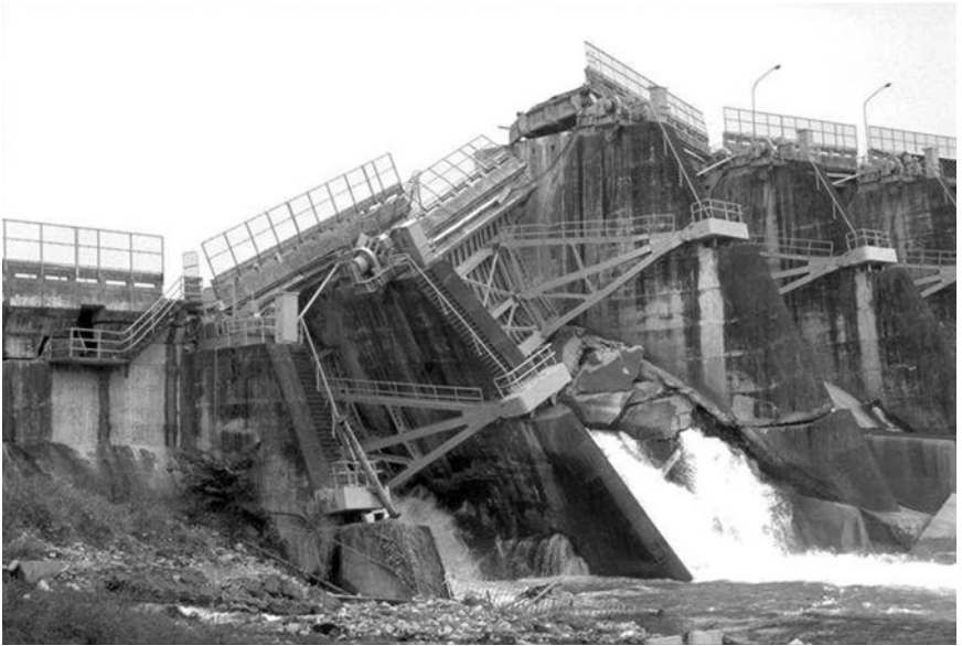
FIGURE 3.4 Close-up view of the location of the dam damaged by surface fault rupture associated with the Chi-chi (Taiwan) earthquake on September 21, 1999. Note in this figure that the entire length of fence on the top of the dam was initially at the same elevation prior to the earthquake. (Photograph from the Taiwan Collection, EERC, University of California, Berkeley.)
