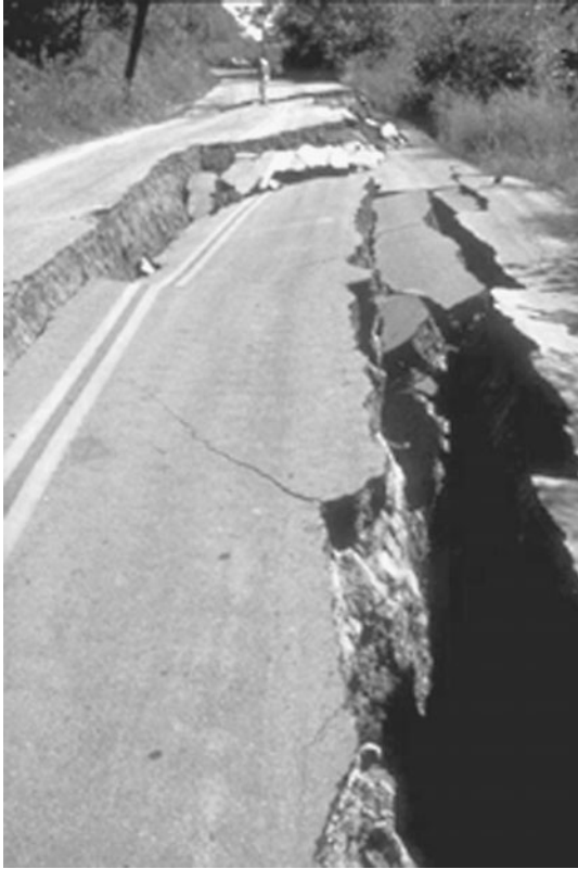
FIGURE 9.34 Earthquake damage to a two-lane road in Santa Cruz Mountains. The slope movement was caused by the Loma Prieta earthquake in California on October 17, 1989. (Photograph from the Loma Prieta Collection, EERC, University of California, Berkeley.)
