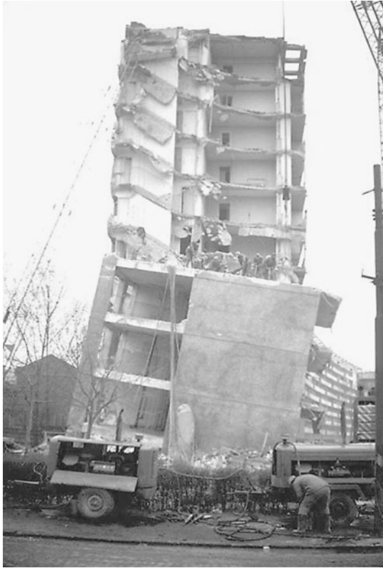
FIGURE 4.19 A comparatively new building that was proclaimed as “earthquake-proof” because of the box-type construction consisting of numerous shear walls. Nevertheless, the structure was severely damaged because of earthquake-induced settlement of the building during the Bucharest earthquake on March 4, 1977. (Photograph from the Steinbrugge Collection, EERC, University of California, Berkeley.)
