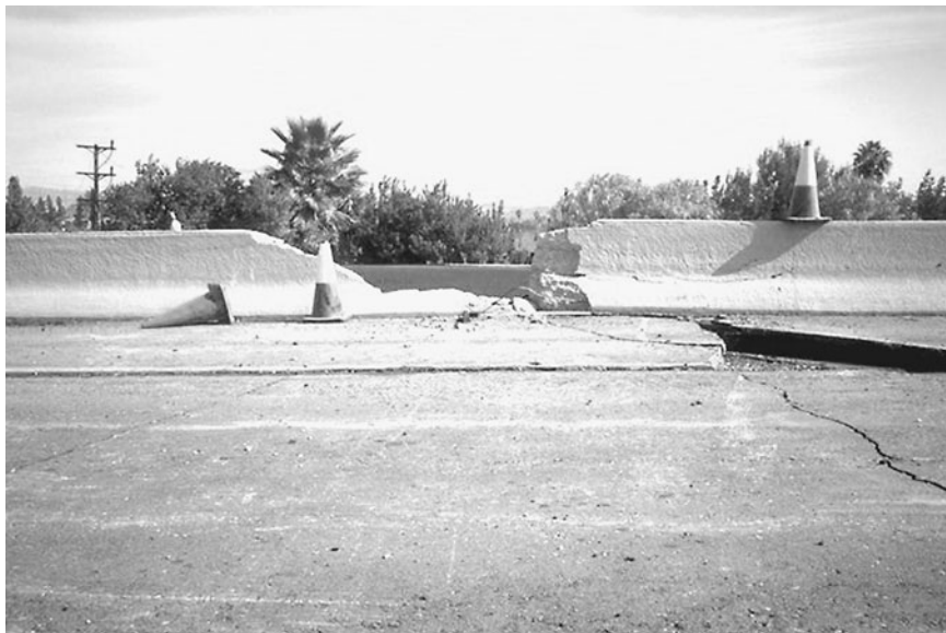
FIGURE 11.4 View to the north along northbound Interstate 405, 250 yards south of Rinaldi Overcrossing. The compressional damage to the roadway and at the median barrier was caused by the Northridge earthquake, in California, on January 17, 1994. (Photograph from the Northridge Collection, EERC, University of California, Berkeley.)
