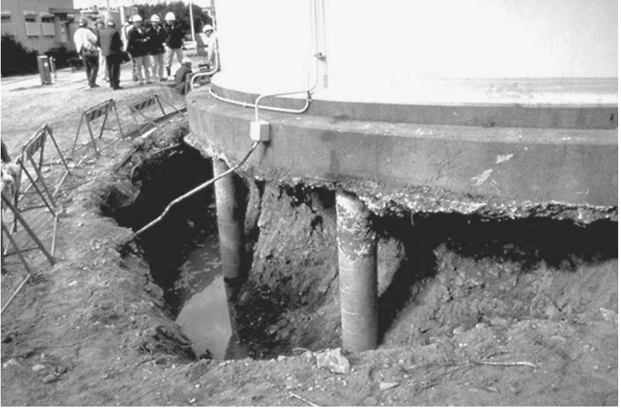
FIGURE 13.5 Storage tank supported by concrete piles. The soil underneath the tank liquefied during the Kobe earthquake on January 17, 1995. The soil around the piles was removed in order to observe the condition of the piles. (Photograph from the Kobe Geotechnical Collection, EERC, University of California, Berkeley.)
