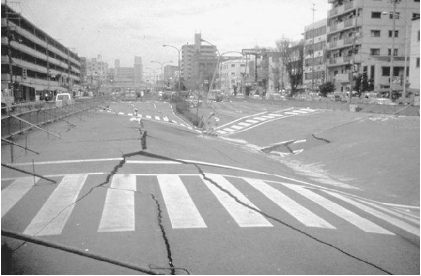
FIGURE 11.7 This picture shows street damage caused by the underlying collapse of the Daikai subway station. The January 17, 1995, Kobe earthquake (moment magnitude = 6.9) in Japan caused this damage. (Photograph from the Kobe Geotechnical Collection, EERC, University of California, Berkeley.)
