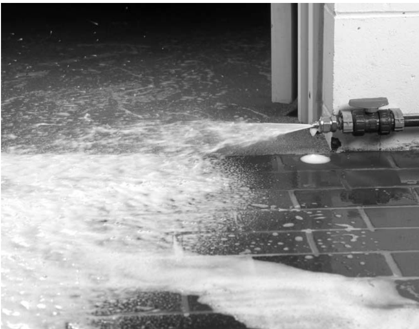
Figure 17-2 Door foaming unit incorporated to reduce contamination from employees and equipment. Courtesy of JohnsonDiversey Inc, Detroit, Michigan.
