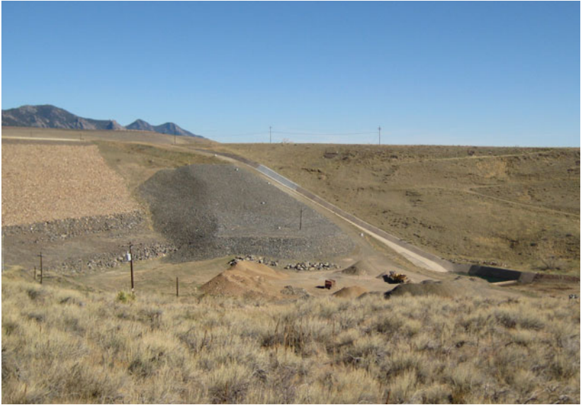
Photo 3. Overview of Ralston Dam left abutment and spillway from the right abutment
