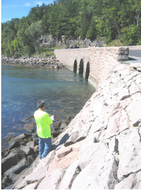
FIG. 6. A structure that grades from slope protection to a bridge approach wall.
