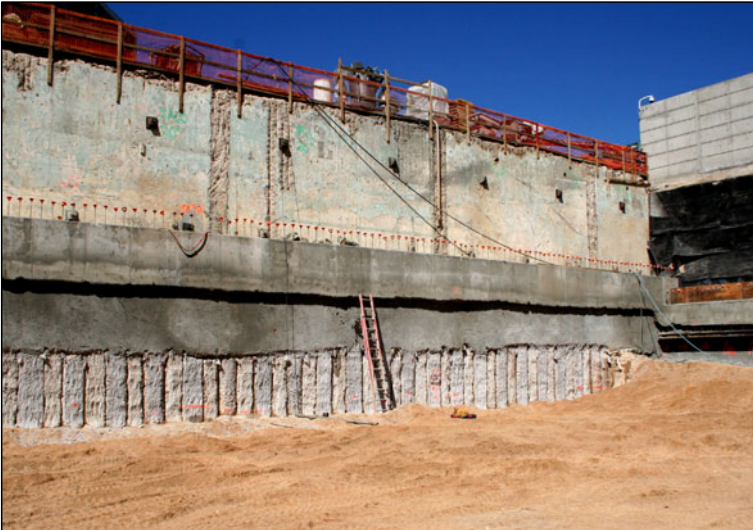
Figure 5: View of postal facility basement and secant walls 3 meters (10 feet) below groundwater elevation (the EPA Building is to the right).
