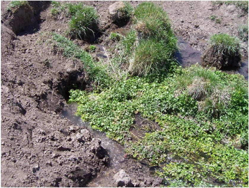
FIG. 6. Surface water entering piping feature in beet spoil slurry deposit, Fort Collins, CO.
