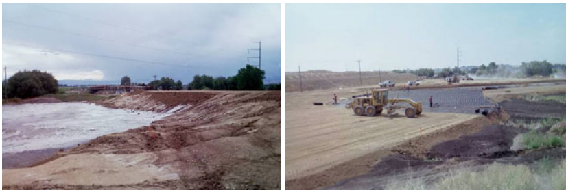
FIG. 7. Construction of roadway embankment over beet spoils and stabilization of subgrade using Geogrid.
