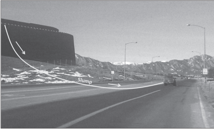
FIG. 5. Rocky Mountain Metropolitan Airport landslide
