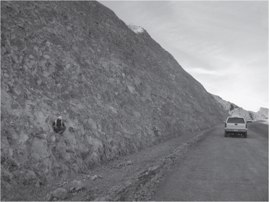
FIG 2. Hand-scaling of a cut after construction to reduce probability of failure (hazard)
