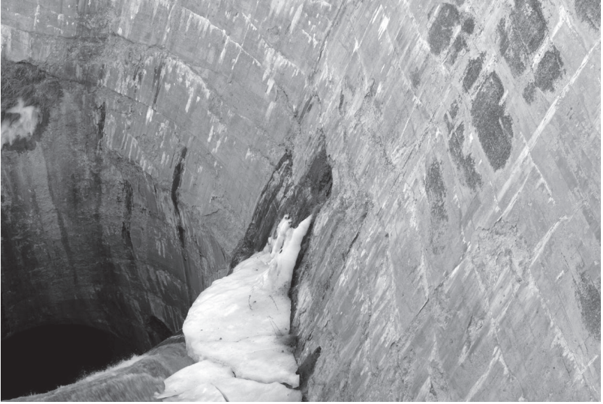
FIG. 2. Freeze thaw damage at the intake
