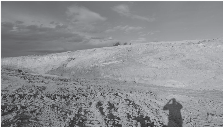
FIG. 4. Silverleaf Subdivision next to the Wildgrass Subdivision, Broomfield, Colorado. Deep excavation of Laramie claystones with sandstone beds and lenses
