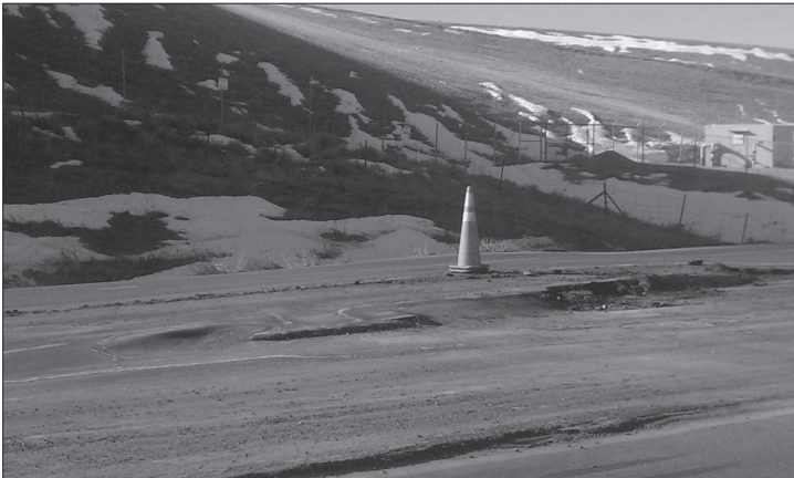
FIG. 6. Toe of Rocky Mountain Airport landslide in State Highway 128
