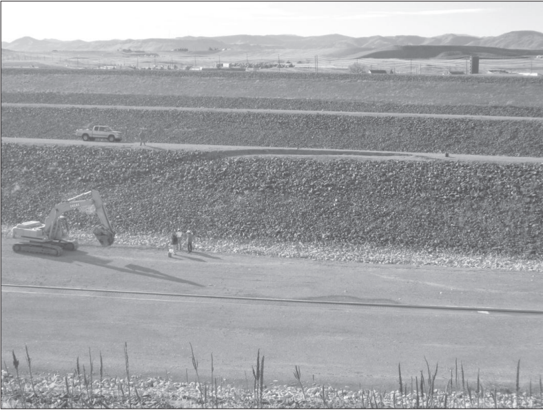
FIG. 9. Laramie claystone landslide on internal dike
