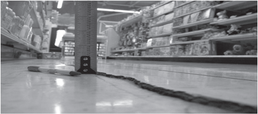
Photo 1: Floor Slab Damage Retail Store
