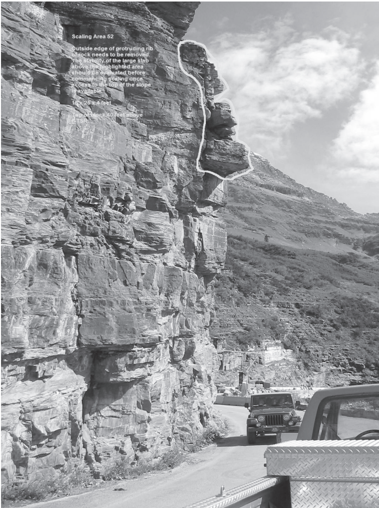
FIG 1. Rock slope at Glacier National Park where rockfall is expected to reach the travel lanes of the road (courtesy of Cornforth Consultants, Inc.)
