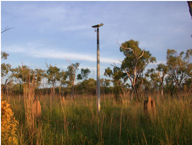
Fig. 7.3 Station mounted on a Tower (Source: Andrew Taylor)
