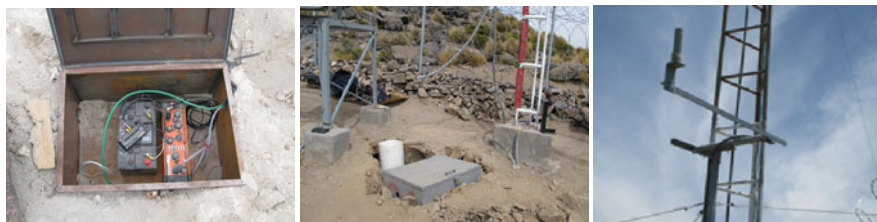
Fig. 2.2 Peru seismic station. From left to right , node hardware internals showing the batteries, digitizer, and node hardware; overall view of the node installation site, including the seismic sensor itself inside the PVC tube; WiFi antenna installation. Original images used with permission of Ing. Victor Aguilar Puruhuaya
