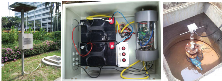
Fig. 2.3 The WaterWise System. From left to right : the node installation with solar panel; a view of the inside of the junction box, showing the batteries, solar charge controller, and the node itself in its watertight packaging; and a tapping point assembly installed inside a manhole, with a electromagnetic flow meter installed during calibration tests. Original images used with permission of Amitsur Preis, SMART Center
