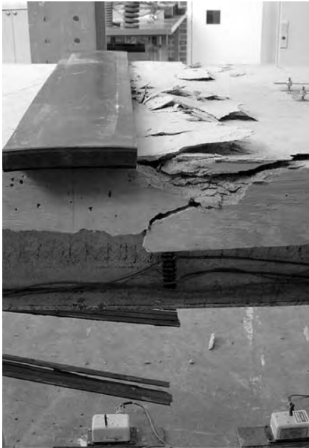
Figure 13. Concrete crushing failure and CFRP strip rupture of steel-concrete composite girder (CGAB-I).
