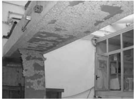
Figure 3. Bottom View of B-2 Beam at Failure.
