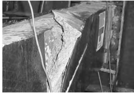
(a) debonding (beam CJE).
