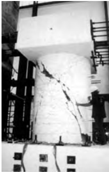
Figure 3. Cyclic load test on full scale bridge pier. The control specimen shows extensive cracking of the RC pier (Fyfe 2001).
