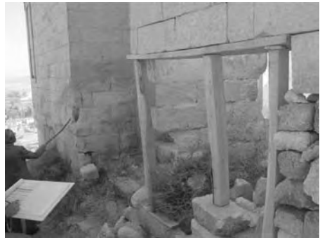
Figure 3. Eroded stones at the slopes.
