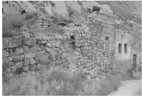
Figure 2. Erosion and dislocation of stones.
