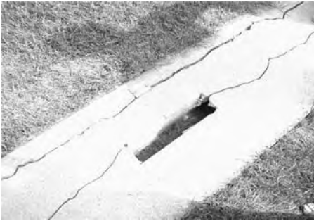
Figure 22. Longitudinal cracking of the pre-stressed hollow beams.
