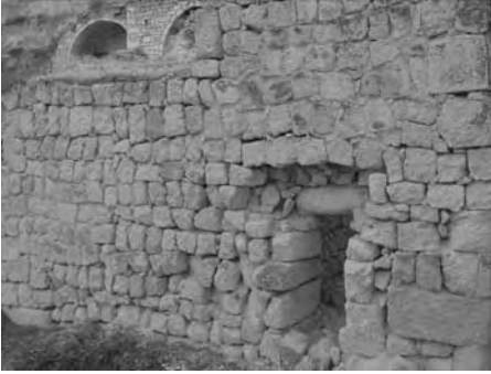
Figure 4. Lost lintels, impending walls for collapse.
