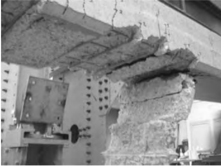
Figure 1. Bottom View of A-2 Beam at Failure.
