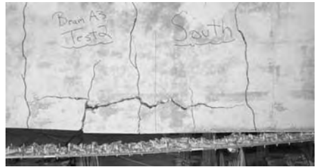
Figure 13. Delamination failure of strip in A3-2.
