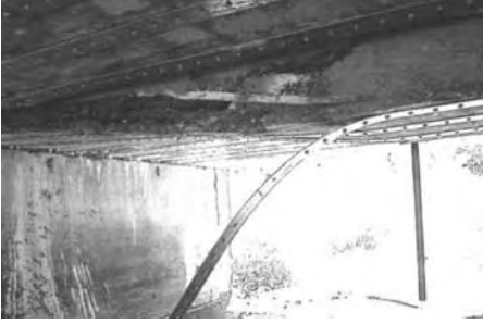
Figure 21. Failure of the West section.
