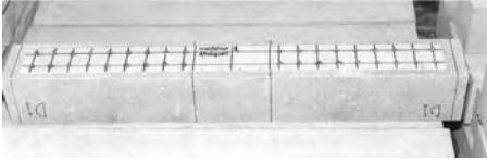
Figure 2. Standard FRP strip attached to underside of 1.2 m beam with powder-actuated fasteners.
