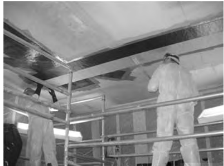
Figure 1. Strengthening before holing of a ventilation shaft in an existing structure due to a changed area of use. Stabilator AB.
