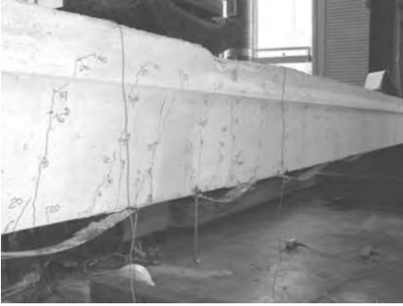
Figure 6. Debonding of externally bonded CFRP strips.
