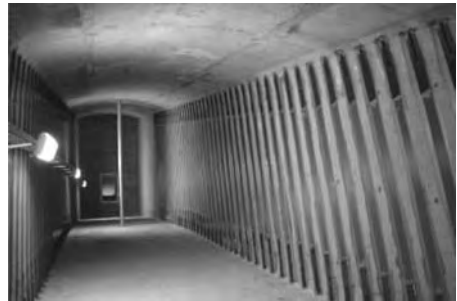
Figure 3. Result after strengthening – seen from inside the bridge. This photo shows strengthening approximately from section A to the column no. 8.
