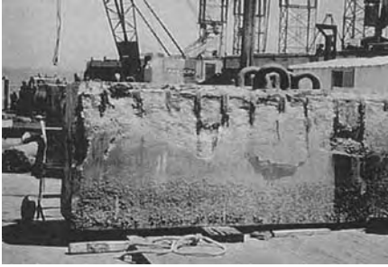
Figure 2. Damaged fender support beam, Qatar (courtesy EUROCRETE project).
