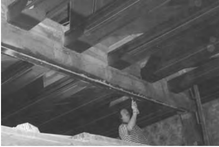
Figure 3. CFRP and polymer concrete strengthening of a historic ceiling joist in waffle slab, Mansfeld castle (D).
