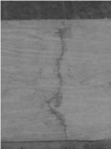
Figure 5. Flexural crack located at the bottom of RC beam.
