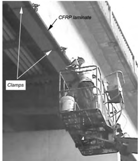
Figure 10. Application of CFRP laminates to the bottom of Girder 5 in Span 6 by a trained worker on a movable crane.
