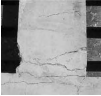
Figure 3. Ultimate failure of specimen CSM0.
