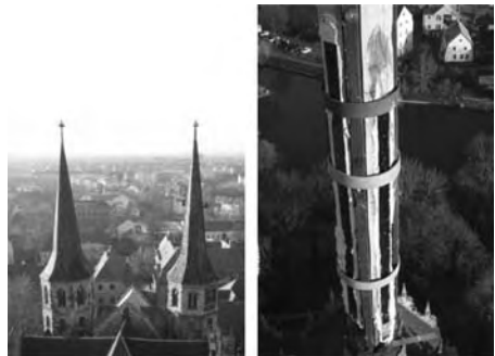
Figures 1–2. Damaged spire of the Merseburg cathedral (D) due to high wind loads and weathering. Cantilever joint after strengthening with CFRPs.
