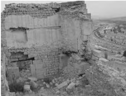
Figure 15. Massive and unstable walls.
