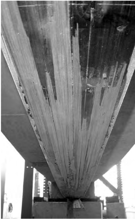
Figure 14. Soffit of girder (CGAB-1) showing interlaminar shear failure of CFRP strip away from midspan.
