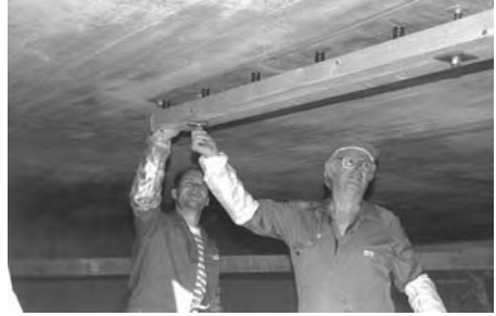
Figure 1. Strengthening of a concrete bridge with steel plates. Carried out in Sweden during the mid 1990s.
