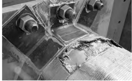
Figure 6. Detail of local buckling at base showing anchorage angles for sheets.
