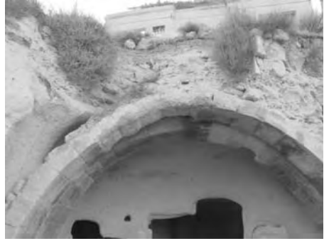
Figure 6. Arch keystone erosion.
