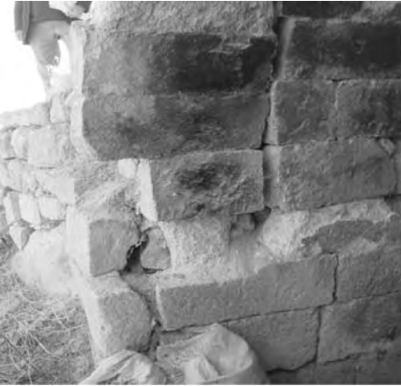
Figure 5. Arch feet erosion.
