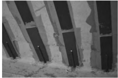
Figure 2. Anchor system for the CFRP laminates. The anchorages are bonded with an epoxy adhesive in pre-drilled holes in the flanges.
