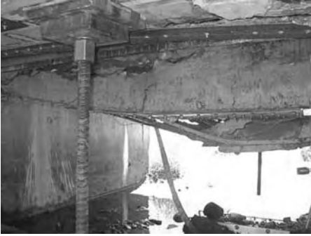
Figure 22. Failure of the East section (foreground) and West section (background).
