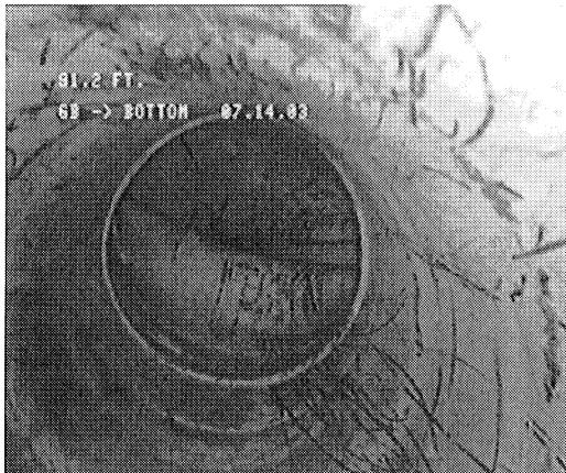
Figure 3. - Distressed elbow in Subcell B riser
