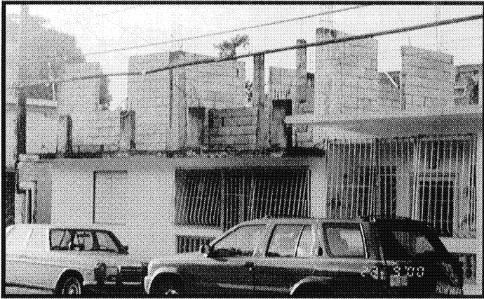
Figure 2. Inadequate anchorage length for columns
