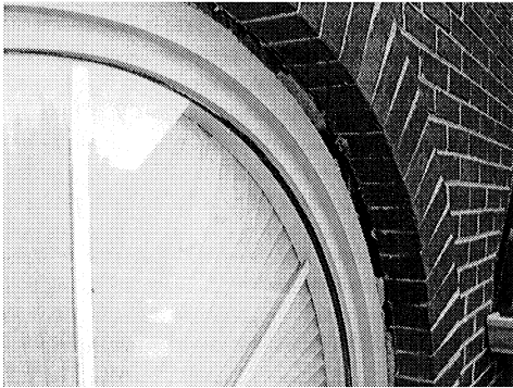
Fig. 3: Gap between curved-head window frame and brick veneer
