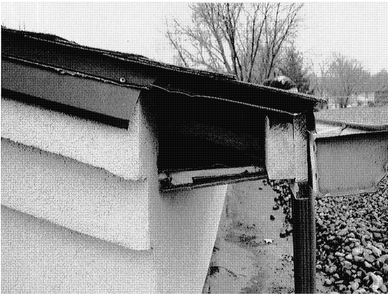
Figure 6 – Open end of soffit at gable eave for sloped roof. The poorly executed fascia extension is also seen at the raked edge of the slope roof.
