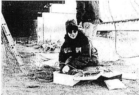
Figure 7. Strain transducer and wind sensors cables installation to the data logger prior to placing into service.
