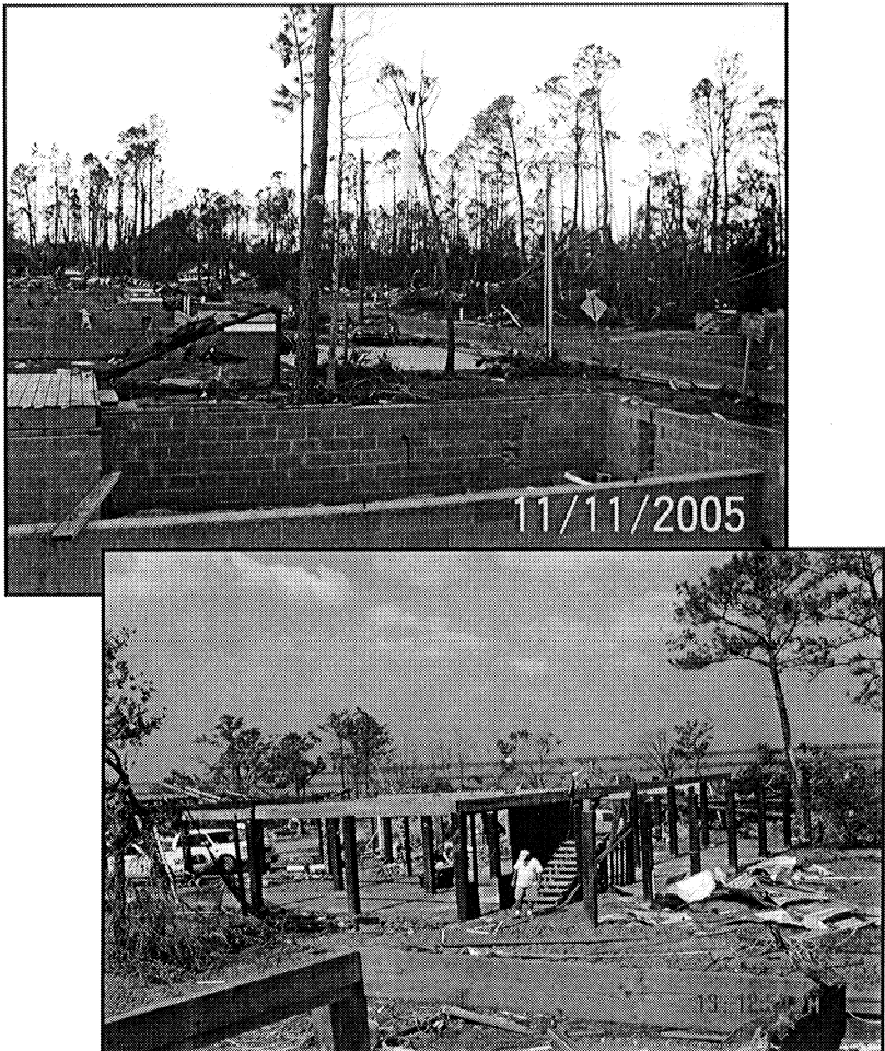
Figure 6: Typical views of devastation along the Mississippi coast caused by Hurricane Katrina. Determining the extent of wind damages prior to the storm surge sweeping through these sites was a daunting task for the structural engineer.
