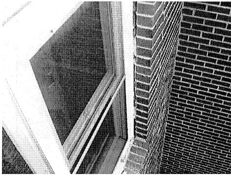
Fig. 2: Gap between window frame and brick veneer
