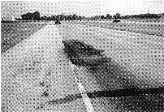
Figure 1 Severe Distress, Section 390103
