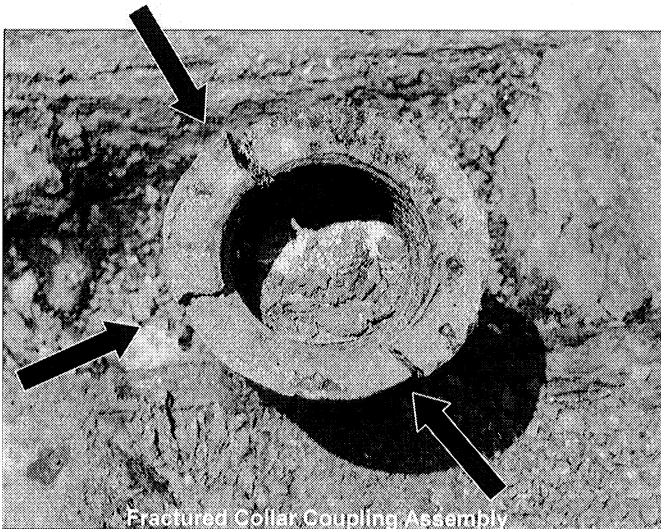
Photograph 3 – Delineating Through-Wall Cracking
