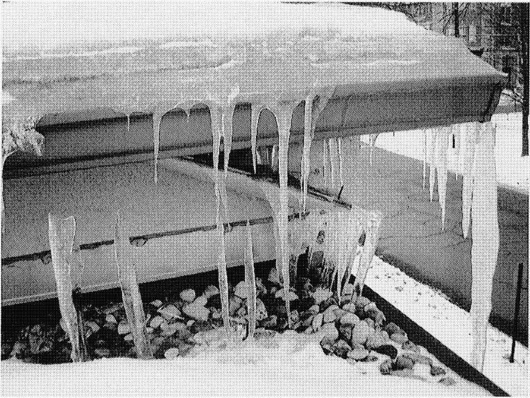
Figure 7. Ice damming at the sloped roof eave.
