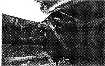
Figure 7. Boarded up tunnel face following the collapse due to running ground at Edgemont Ave.
