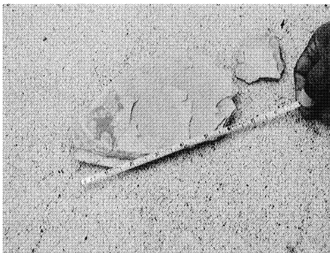
Figure 5. Piece of delaminated limestone measures 7" in length.
