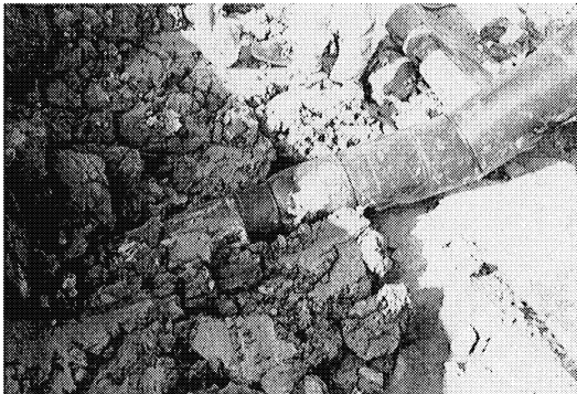
Figure 6. - Condition of bedding soil around elbow
