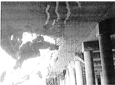
Fig 3. Collapse along existing cracks
