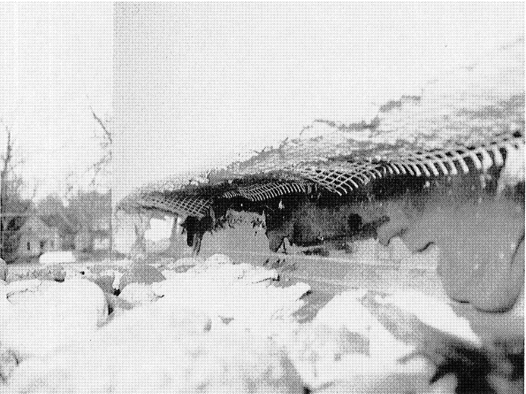
Figure 4. EIFS system is improperly terminated without backwrapping.
