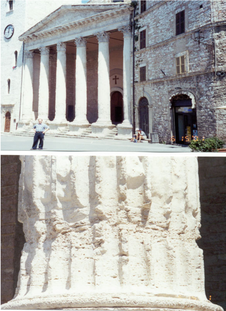
Fig. 13.2 Biodeterioration of the columns of ancient Roman temple caused by nitrifying bacteria
