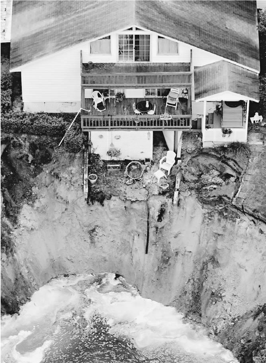
A home in Lake City, Florida, on the edge of a sinkhole, March 3, 2005. Lowering of the groundwater table has caused many sinkholes to form in southern Florida in recent years. (AP)
