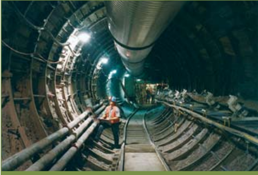
A 1.7-mile (2.7 km) long tunnel used for scientific studies in the potential high-level nuclear waste repository at Yucca Mountain, Nevada. (U.S. Department of Energy)
