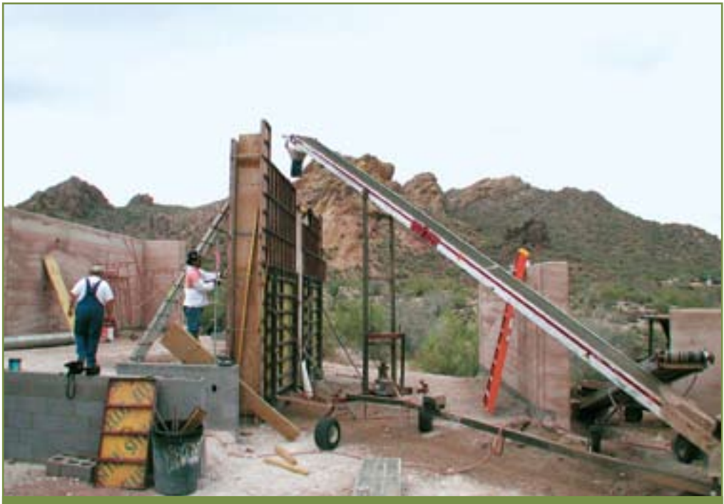
Construction on a rammed earth house outside Phoenix, Arizona. The thick rammed earth walls provide insulation from the desert heat. ( James Elser )
