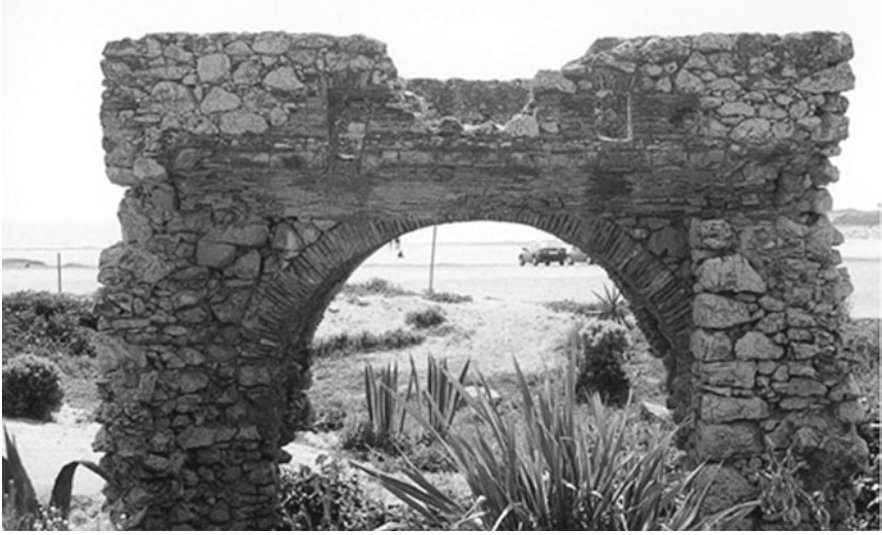
Fig. 11 Note the holes in the wall of the pond room prepared for two waterwheels. From the information available, only one wheel and one set of millstone were installed
