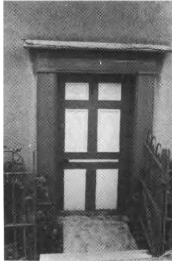
Figure 5.1 Settlement on peat at Benwick, Hunts. The entrance to the house has settled by about 1 m below pavement level
