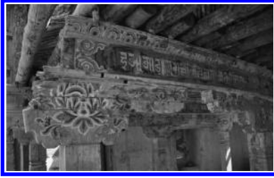
Figure 2. Broken beam mount.
