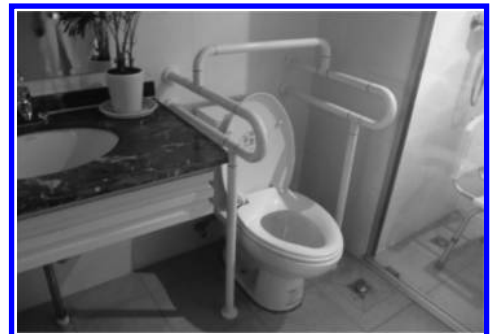
Figure 3. Safety handrail on toilet.
