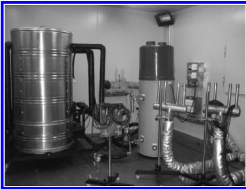
Figure 2. Experimental set up air source heat pump.
