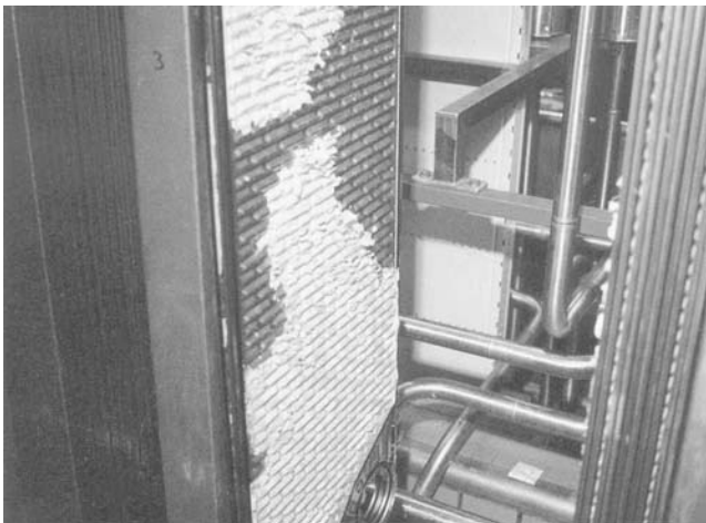
Fig. 1.9 Fouled plate of a heat exchanger after processing milk.
