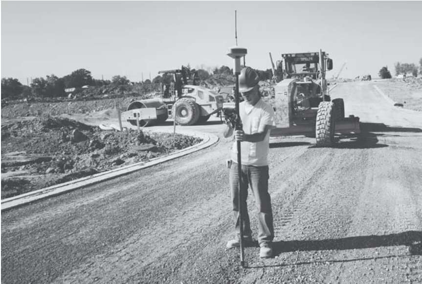
Figure 14.1 GNSS receiver being used in a construction site. (Courtesy Topcon Positioning Systems.)
