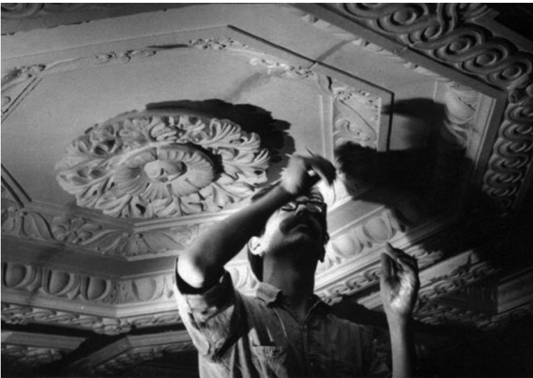
Figure 7 Author installing an ornamental plaster ceiling, Wilkes Barre, Pennsylvania, while employed at Felber Studios, Horsham, Pennsylvania. 1970. Source: Photograph courtesy of author’s archives.
