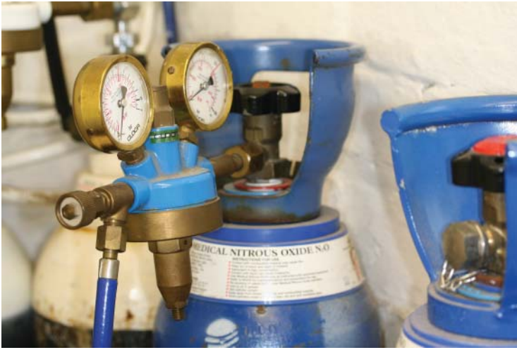
Figure 13.9 Nitrous oxide tank, valve and gauge
