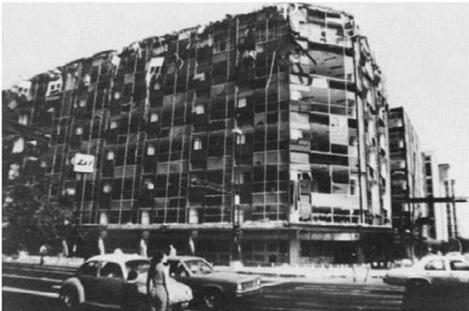
Figure 11.31 Large-scale damage in the upper floors of a flexible building, Mexico City, 1985.
