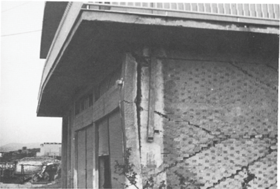
Figure 11.8 Damage in column in contact with masonry on one side only, Loutraki, Greece, 1981.
