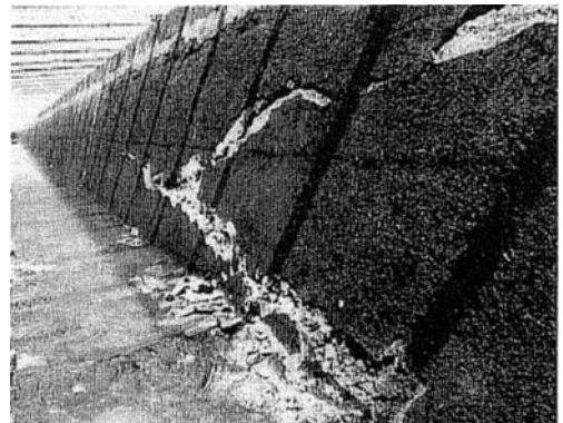
Photo.6 Damage of Side Wall of In Take Channel
