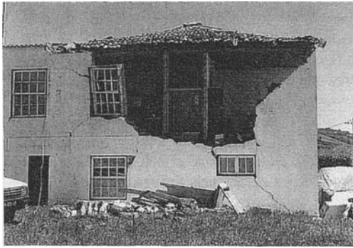
Figure 5. Typical damage at zones 15 km from the epicenter to block masonry houses; amplification due to soil layers.
