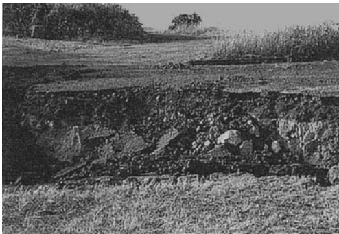
Figure 6. Differential soil settlement at road side on top of hill.
