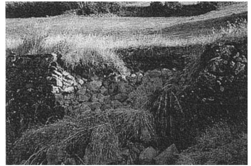
Figure 8. Collapse of road retaining wall.
