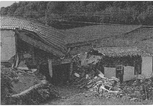
Figure 4. Typical damage at zones 5 to 10 km from the epicenter to rural houses of rubble masonry and to houses with some reinforced concrete beam elements.
