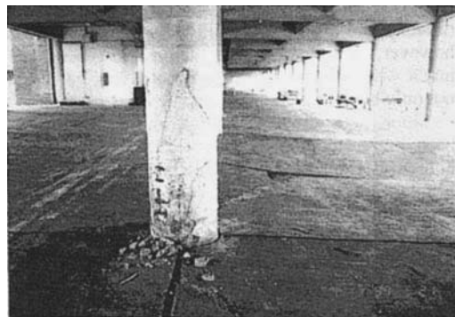
Figure 13 Damage to column and differential settlement of ground
