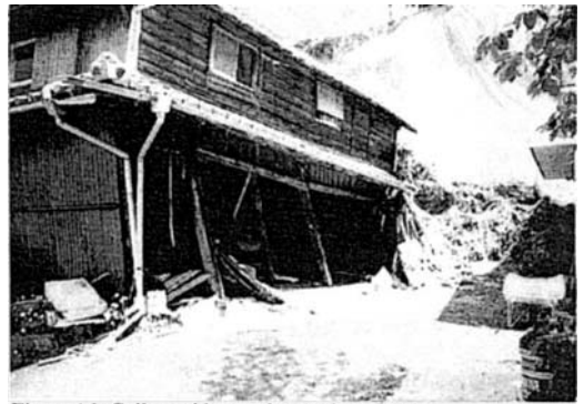
Figure 16 Collapsed house due to slope failure
