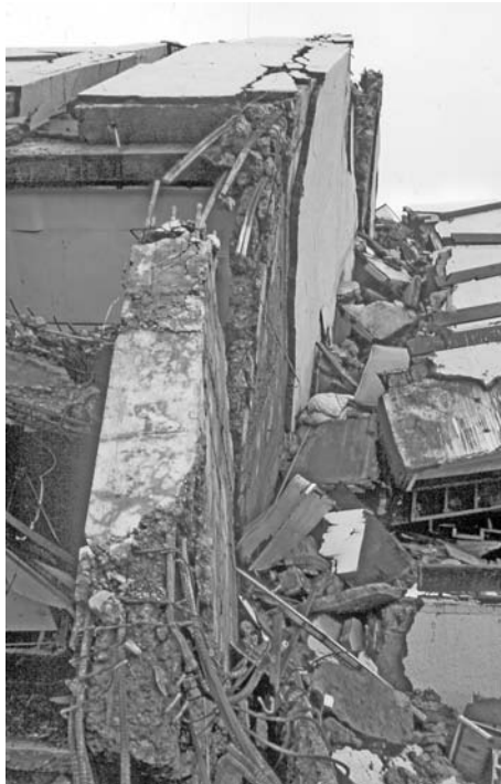
Fig. 1.20 Collapse of tall shear wall building, Baguio, Philippines, 1990
