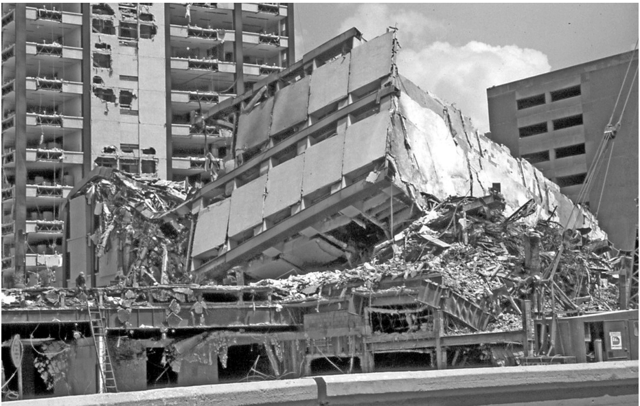
Fig. 9.1 Collapse of Pinot Suarez building, Mexico City, 1985
