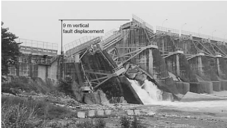
Fig. 1.2 A fault passed through the Shinkhang dam, Taiwan, in 1999, causing the vertical displacement of 9 m
