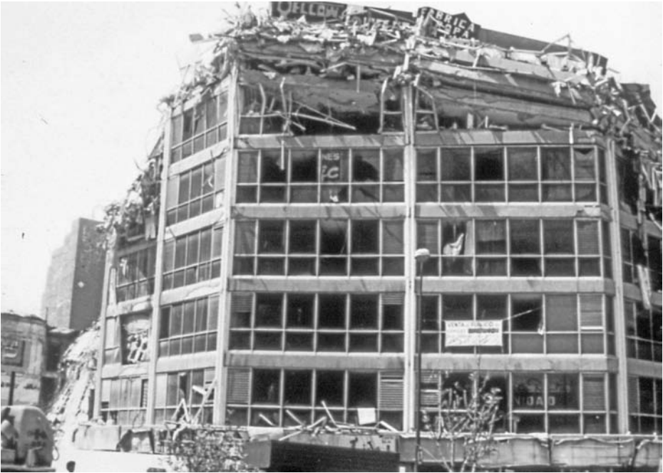
Fig. 1.6 Upper-storey collapse of a multi-storey reinforced concrete structure in Mexico City, 1985
