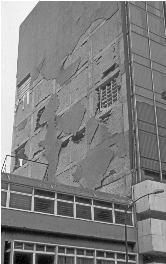
Fig. 12.1 Failure of a ‘displacement-sensitive’ non-structural element: façade cladding Mexico City, 1985
