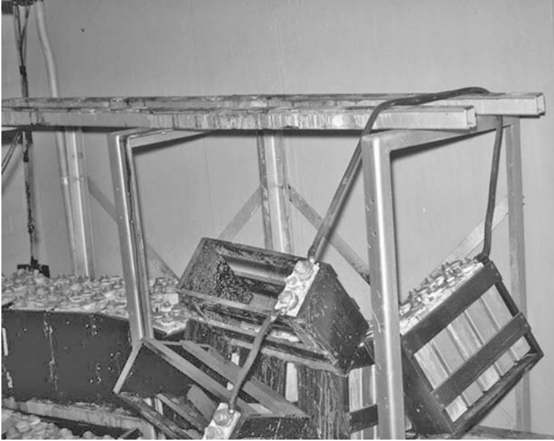
Fig. 1.13 Earthquake damage to internal fixings has caused batteries to fail in a hospital in San Fernando, USA, 1971
