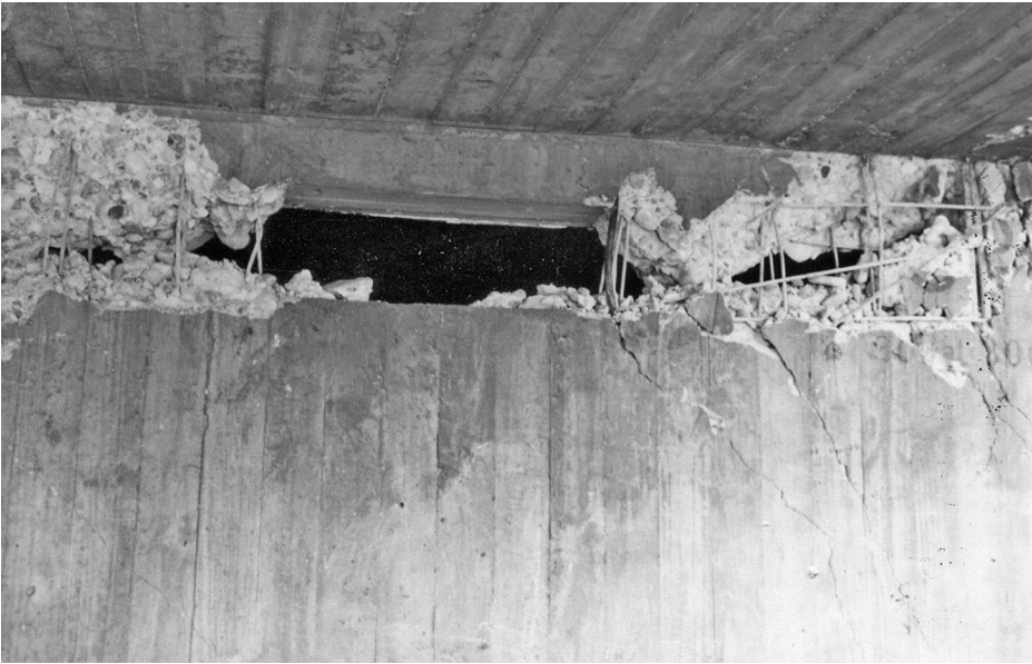
Fig. 8.20 Damage around opening in a shear wall, 1985 Chile earthquake
