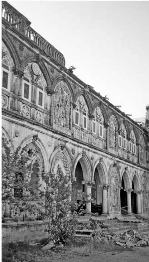
Fig. 1.12 Parapet failure, Gujarat, India, 2001
