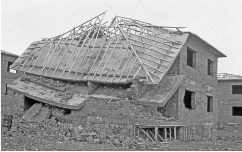
Fig. 1.10 Failure of modern clay brick house in Erzincan, Turkey, 1992
