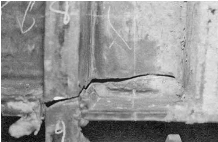
Fig. 9.2 Brittle failure of steel structure in the Northridge, California earthquake of 1994
