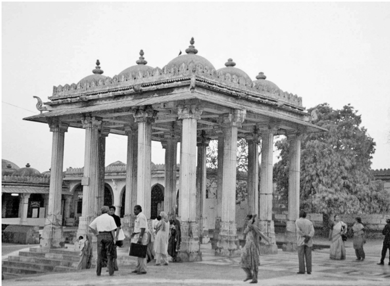
Fig. 10.7 Response of masonry columns supporting a heavy masonry roof slab, Gujarat, India earthquake, 2001. The columns of this ancient structure, which were unreinforced, showed some cracking but survived an earthquake which toppled many modern reinforced buildings in the Indian city of Ahmadabad
