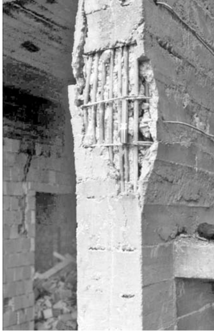
Fig. 1.19 Compression failure of outside edge of shear wall, Erzincan, Turkey, 1992
