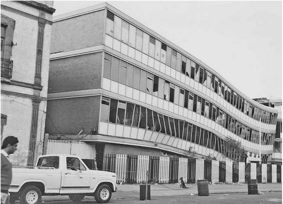
Fig. 1.8 The nearer end of this building is restrained by stiff shear walls but the far end was supported by slender columns. The resulting torsional movement has led to collapse in Mexico City, 1985
