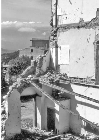
Fig. 1.14 Failure to tie in floor joists to walls probably precipitated failure in this housing in the Friuli, Italy earthquake, 1980
