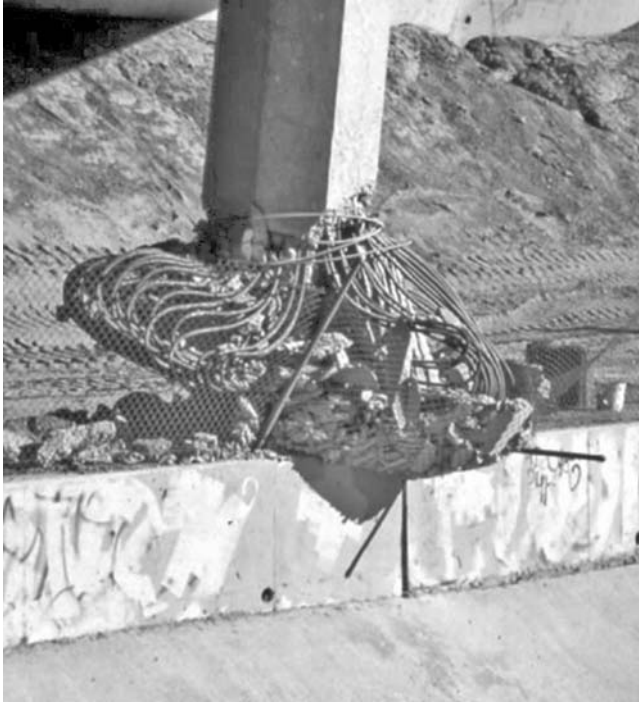
Fig. 1.16 Bursting failure in a column, Northridge, California, 1994. Inadequate horizontal steel has caused the heavy main bars to buckle, and allowed the concrete in the column to shatter
