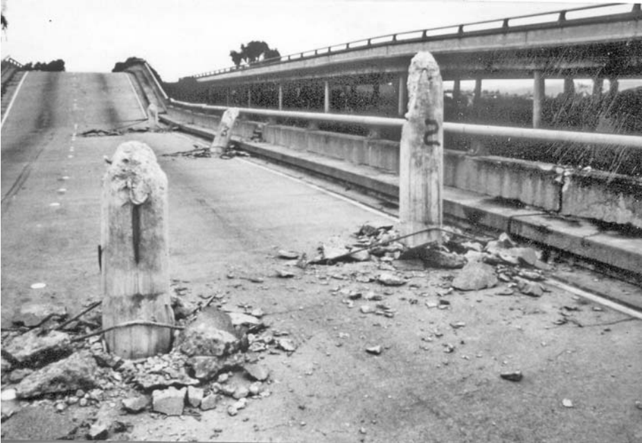
Fig. 1.24 Failure at pile-superstructure in a bridge, Loma Prieta earthquake, California, 1989
