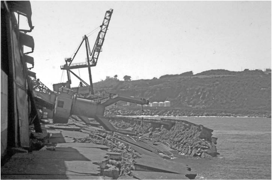
Fig. 7.6 Failure of a quay wall, San Antonio, Chile, 1985
