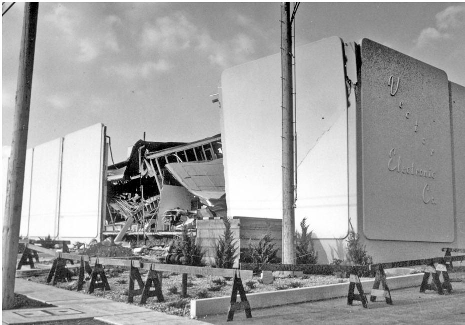
Fig. 8.22 Failure of tilt-up warehouse building, Loma Prieta earthquake, California, 1989
