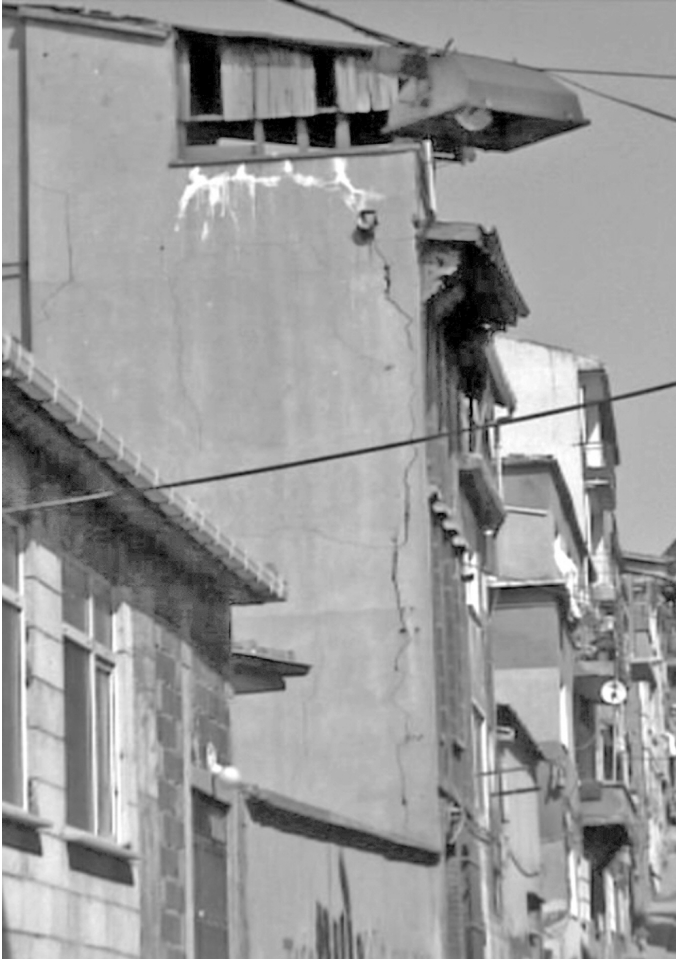
Fig. 10.5 Overturning failure of a façade in a historic masonry building
