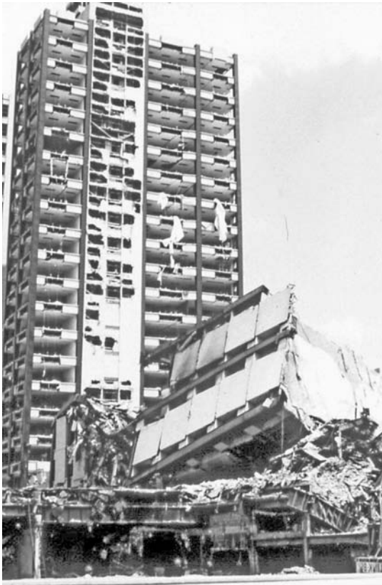
Fig. 1.11 Failure of multi-storey steel-framed buildings, Mexico City, 1985
