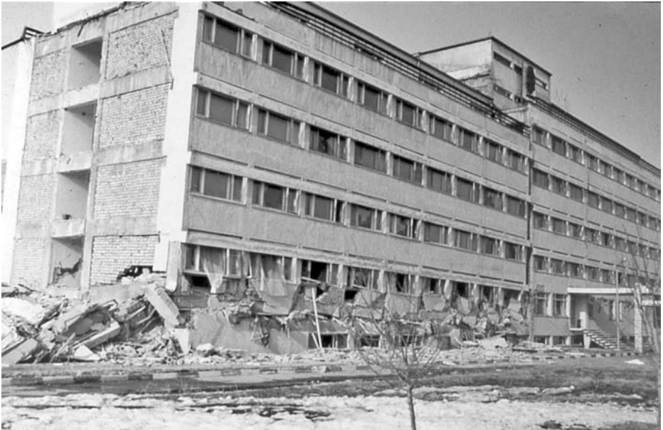
Fig. 1.4 Ground-storey (soft-storey) collapse of buildings in Erzincan, Turkey, 1992
