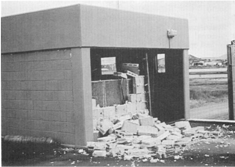
Fig. 1.22 Out-of-plane failure of an unreinforced, unsecured masonry panel, Antigua, 1974
