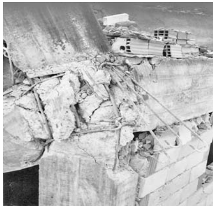
Fig. 1.15 Failure of a beam–column joint in Erzincan, Turkey, 1992. Note failure of the concrete in the joint, and bursting out of column steel
