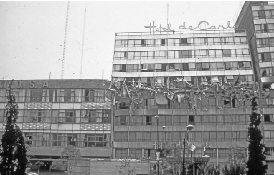
Fig. 1.7 Intermediate-storey failure of a multi-storey structure in Mexico, 1985, probably caused, or aggravated, by buffeting against the adjacent building
