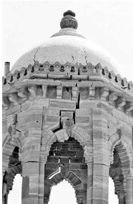
Fig. 1.21 Damage to a palace after the Gujarat, India earthquake of 2001
