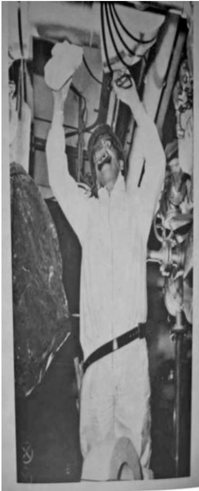
Figure 23-2. A workman removing insulation containing asbestos shows cavalier lack of caution. He should be protected with an air supply respirator venting into his impervious clothing and gloves. He must gather all material into double thickness strong plastic bags for safe disposal.
