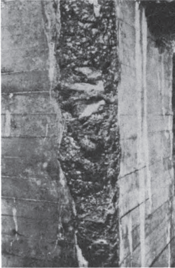
Fig. 9.16 Frost attack, Glenfinnon Viaduct.
