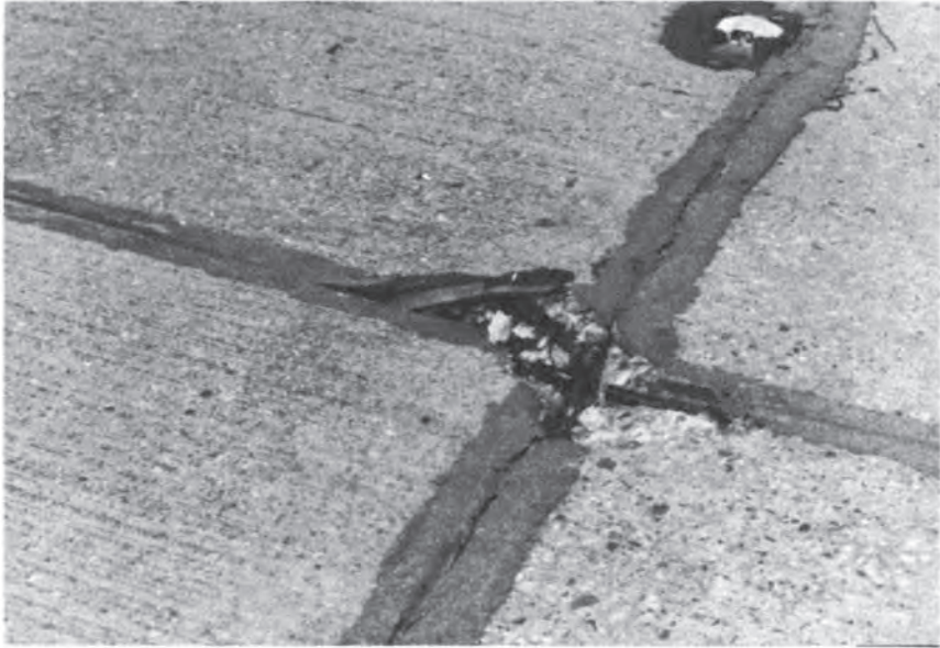
Fig. 10.11 Ineffectiveness of overbanding
