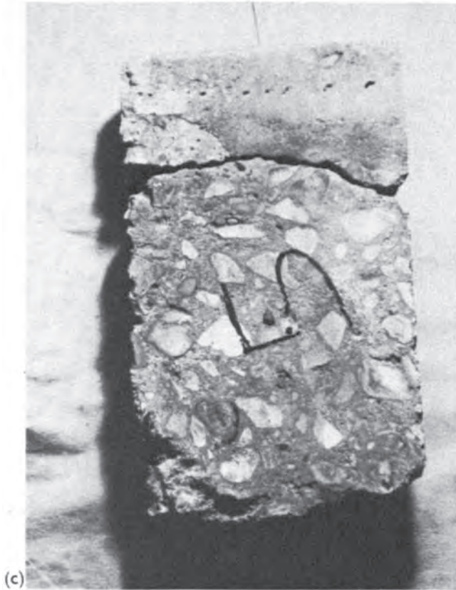
Fig. 5.16 Cores extracted in 1983 from a 1930s reinforced concrete factory building: (a) uncoated concrete from interior surface; (b) concrete coated in 1952; (c) core from an area repaired with mortar and coated in 1952. The cores have been sprayed with phenolphthalein solution; lighter areas indicate depth of carbonation. (Courtesy of W.J.Leigh & Co.)
