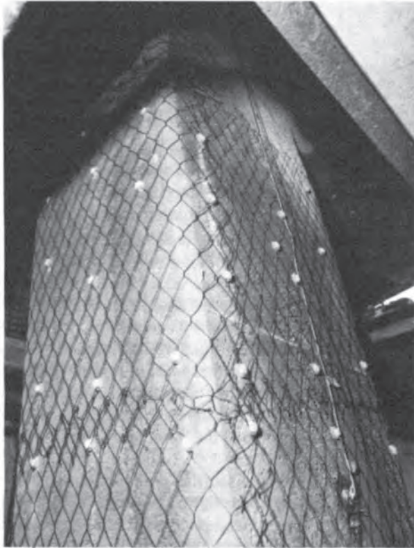
Fig. 5.10 Metal oxide ('chicken wire') mesh fixed to bridge column (courtesy of ICI Chemicals & Polymers, Runcorn, Cheshire).
