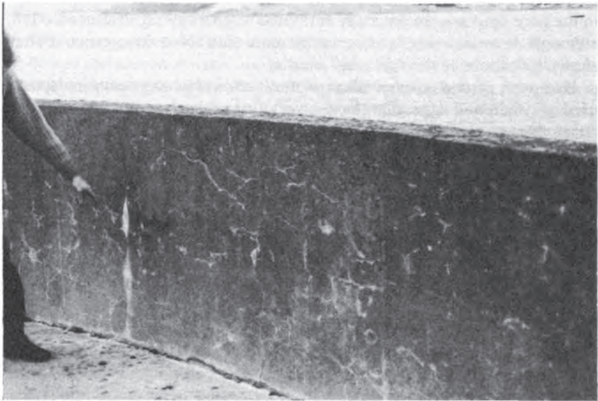
Fig. 2.8 Unrestrained map cracking on parapet wall due to alkali-silica reaction.
