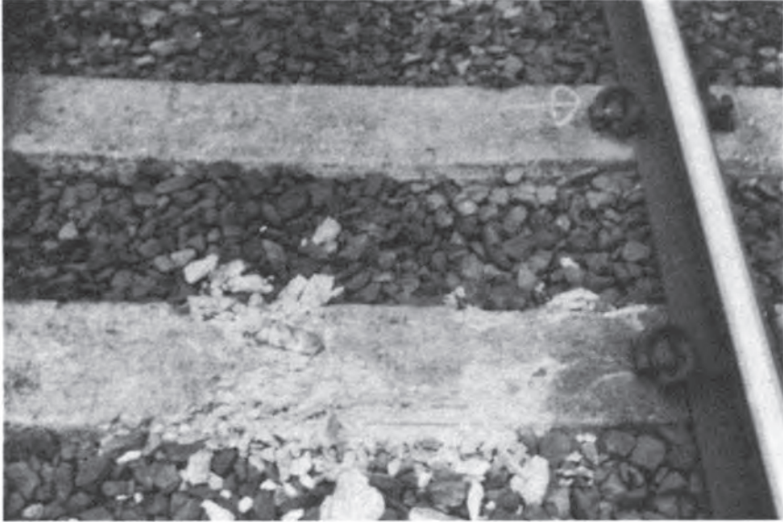
Fig. 9.15 Frost attack, prestressed concrete sleeper.
