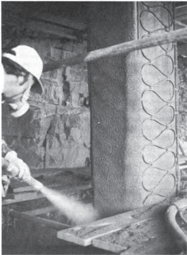
Fig. 5.6 Fixed anode cover coat on bridge column (courtesy of Raychem Ltd, Swindon, Wilts.).
