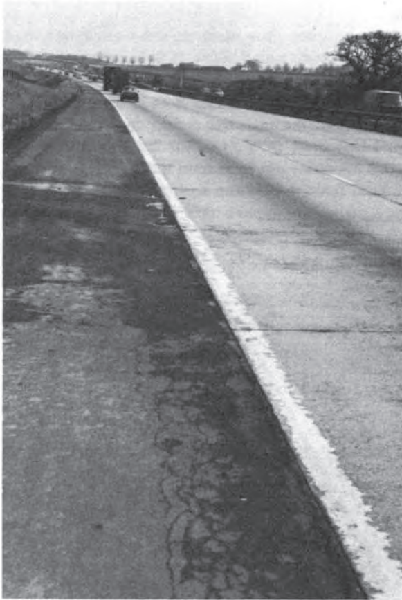
Fig. 10.5 Seepage of water over the hard shoulder from beneath the concrete carriageway.
