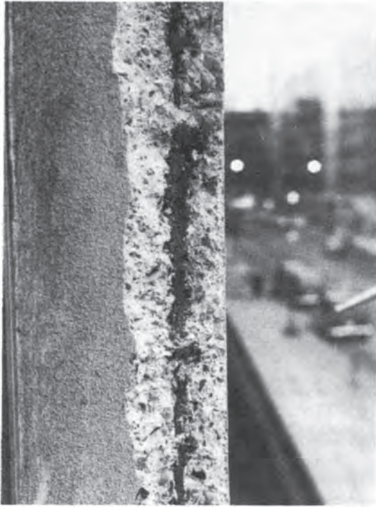
Fig. 9.13 Repair failure on multistorey office block, London.
