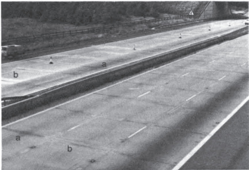
Fig. 10.6 Slip-formed concrete pavement: a, poorly compacted permeable concrete at transverse joints in outer lanes; b, joint arris repairs to most transverse joints in centre and inner lanes.
