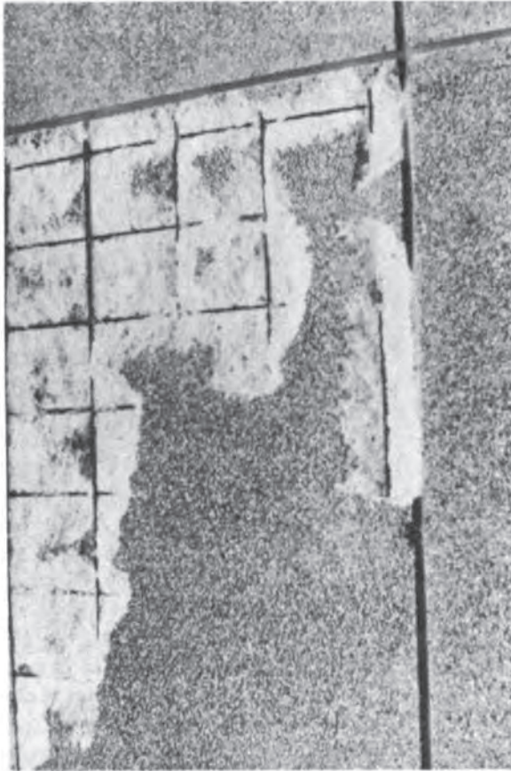
Fig. 9.14 Carbonation at Banbury Station.
