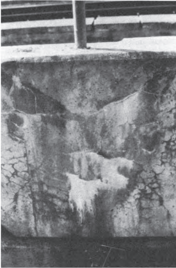
Fig. 9.17 Bridge parapet suffering from alkali-silica reaction.
