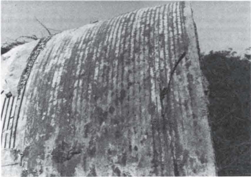
Fig. 5.9 Stray current attack causing premature failure of prestressing wires on concrete pipe.
