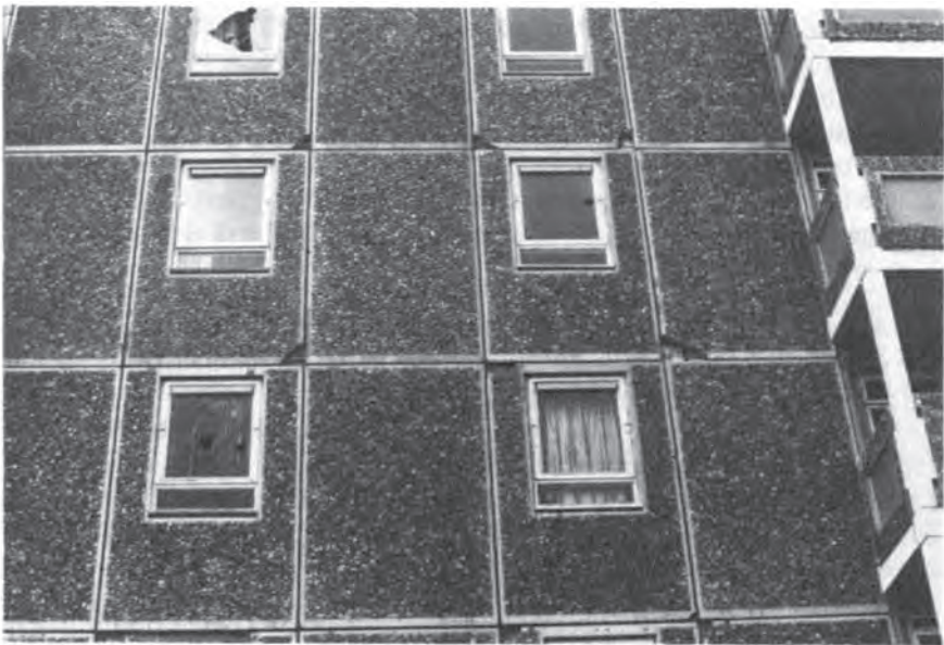
Fig. 7.3 Failure of cladding units at Herbert Willig House
