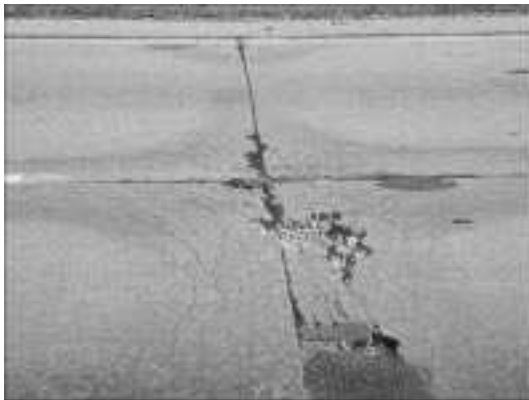
7.1 D-cracking in concrete pavement.
