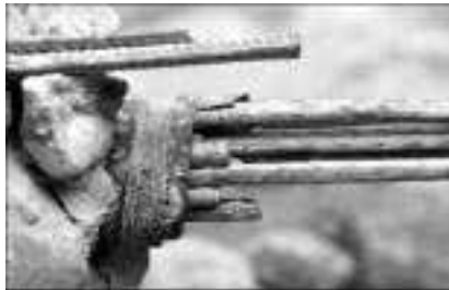
6.14 Broken beam as a result of stress corrosion cracking. Top: survey. Bottom: broken tendon.
