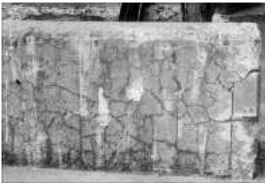
7.3 Map-cracking of concrete wall affected by ASR.
