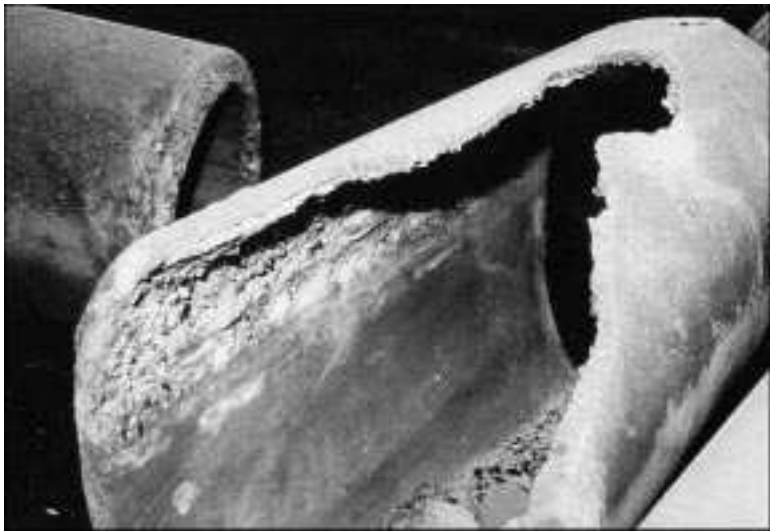
4.4 Microbiologically-induced corrosion in a prefabricated sewer pipe (Case History 11.08.17.01 – reprinted with permission of Elsevier from Corrosion Atlas , 1997, compiled by Evert D.D. Doring).
