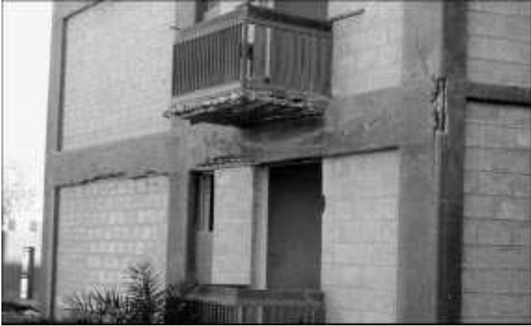
5.1 Reinforced concrete building made with salt-contaminated concreting materials showing effects of reinforcing steel corrosion (Bahrain, circa 1980).
