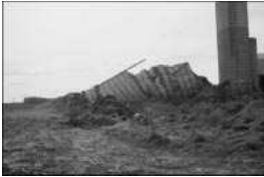
4.5 Collapsed concrete silo showing effects of acid attack (Queen's Printer for Ontario, 1990. Reproduced with permission).
