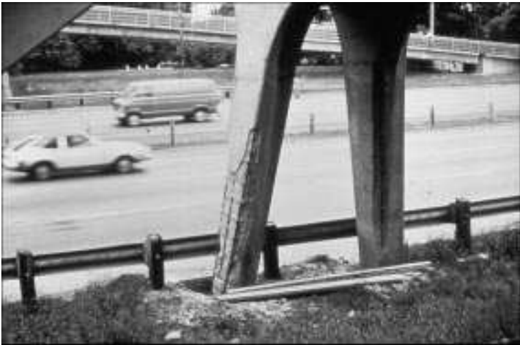
5.2 Reinforced concrete bridge splashed with water containing deicing salt showing effects of reinforcing steel corrosion (USA, circa 1980).
