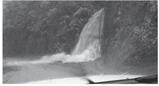
Plate 1. Uncontrolled surface drainage impacting roads.
