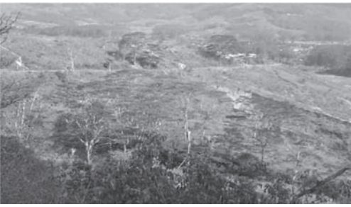
Plate 5. Instability beneath road, Aileu Formation.
