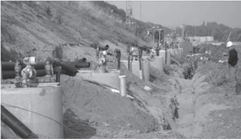
Figure 6. Installation of the vertical extraction wells for the groundwater lowering during active dewatering.
