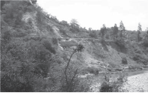
Plate 4. Viqueque formation: gabion wall failure above river.
