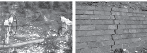
Figure 21. Structural damage after talus slide: damaged bridge piers (left) and crack in retaining wall (right) (Liu 2011).
