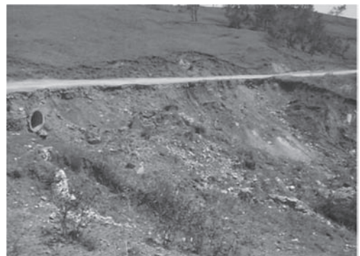
Plate 3. Borbanaro complex: Instability above and below road.
