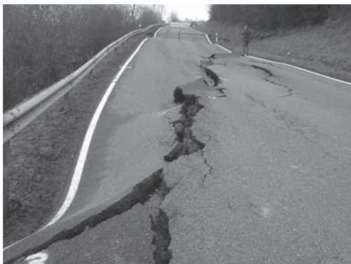
Figure 1. Landslide at the federal road B407 near Kirf.
