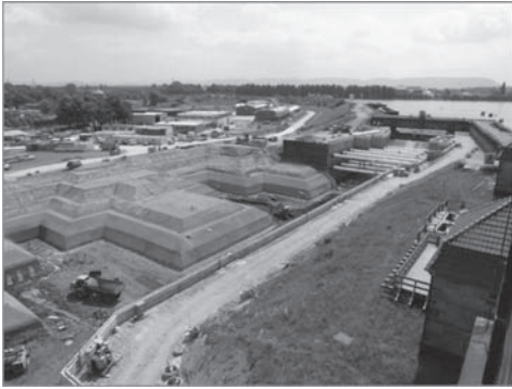
Figure 13. Aerial view of the pit for the new ship in Minden at the final excavation stage.
