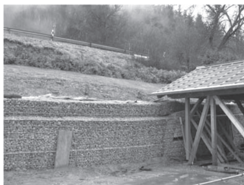
Figure 3. Pushed-over gabion wall at toe of slope near House No. 16.
