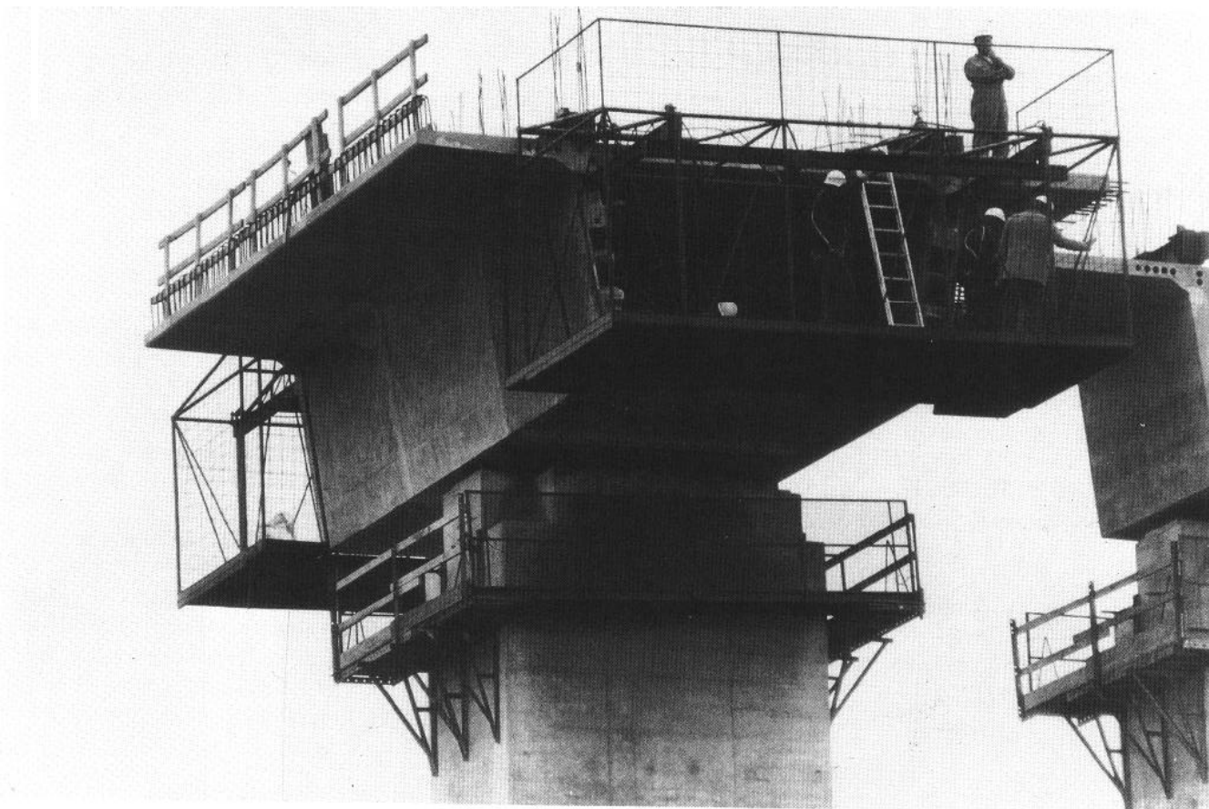
Construction of precast concrete box girder bridge (photo courtesy of Texas Highway Department)
