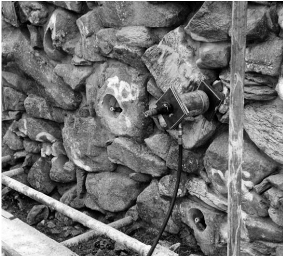
7.35 Epoxy soil nails for retaining wall stabilization, Nant Ffrancon wall stabilization, A5 Trunk Road, North Wales (courtesy of Minova Weldgrip Ltd).
