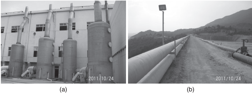
16.16 Extensive uses of FRP vessels and pipelines at Zijin Mining Group, China.
