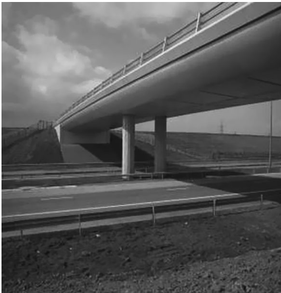
7.17 GFRP bridge enclosure to soffit of approach bridge, Second Severn Crossing (Maunsell Structural Plastics).
