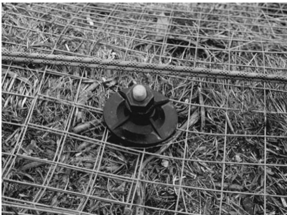
7.33 GRP soil nail and netting, A638 near Wakefield, Yorkshire, UK (courtesy of Minova Weldgrip Ltd).
