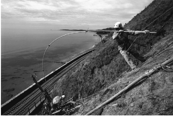
7.34 Installation of GRP soil nails and rock bolts, Dawlish cliff face stabilization, Devon, UK (courtesy of Minova Weldgrip Ltd).
