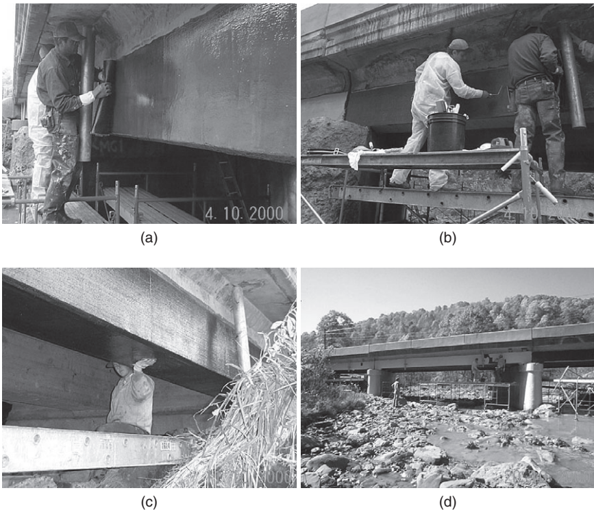
16.22 Rehabilitation of T-section reinforced concrete superstructure using carbon FRP wraps, Muddy Creek Bridge, Preston County, WV (October 2000): (a) blue primer coating and wrap application; (b) pressing of wrap for full bond with concrete; (c) carbon wrapped concrete beam; (d) gray paint application.
