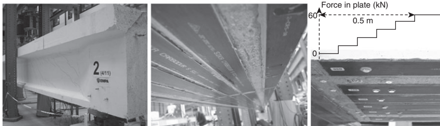
5.8 Full-scale prestressed girder strengthened through bonding prestressed FRP plates using the gradient method to eliminate stress concentrations at the plate ends (Photos taken by the author at EMPA, Switzerland).
