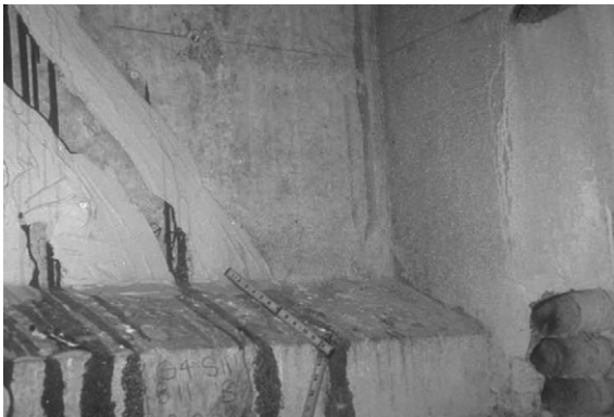
4.19 Some preliminary repair implemented by injecting polyurethane foam in the cracks is seen to be ineffective at I-565 Highway bridge girder in Huntsville.
