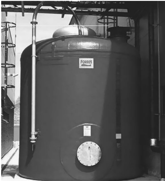
7.23 GRP storage tank (courtesy of Forbes Technologies).
