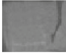
(a) Local image of clevis with a crack
