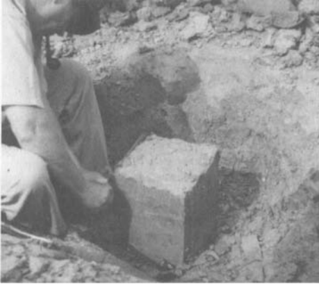
Undisturbed sample being taken from a manually excavated test pit. (Photo courtesy of U.S. Army Corps of Engineers)
