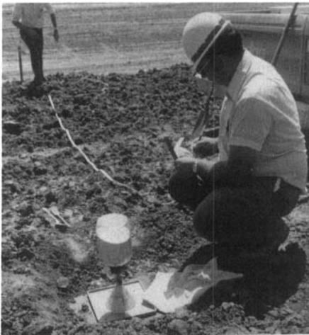
Sand Cone test for in-place density of a fill area. (Photo courtesy U.S. Army Corps of Engineers)
