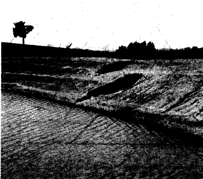
Figure 8.1. Examples of piping failure of a dam due to the presence of dispersive soils (Soil Conservation Service of NSW).
