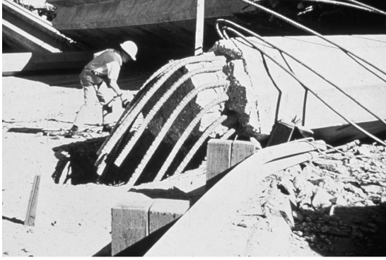
FIGURE 1.13 Lap-splice failure. (With permission from Caltrans.)
