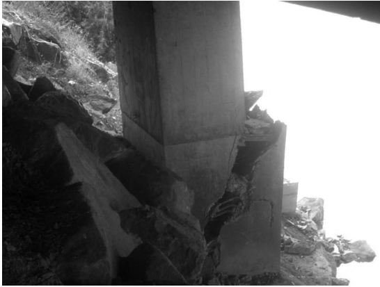
FIGURE 1.14 Column shear failure. (From Chile Earthquake, February 27, 2010.)
