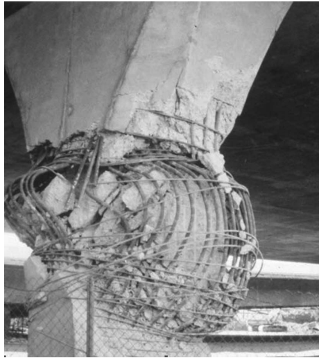
FIGURE 1.11 Compression failure of confined concrete. (With permission from Caltrans.)
