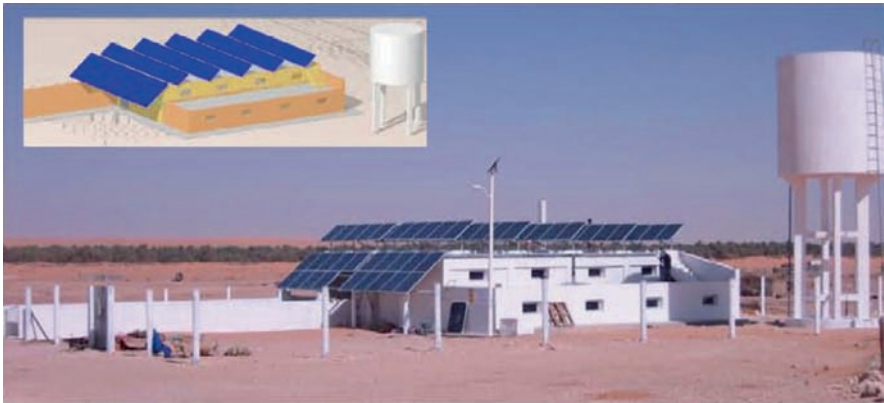
Figure 8.12. Schematic view and photo of the Ksar Ghilène photovoltaic power station and treated water tank.
