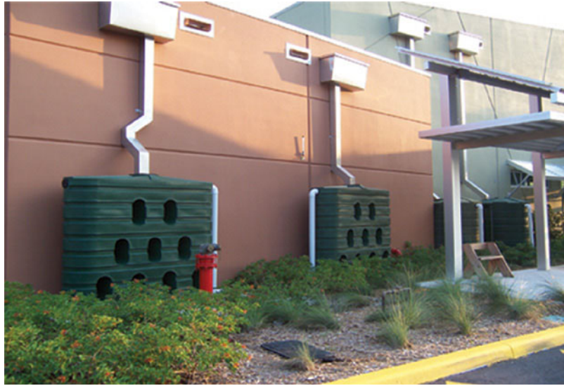
Figure 7.11 School rainwater harvesting project
