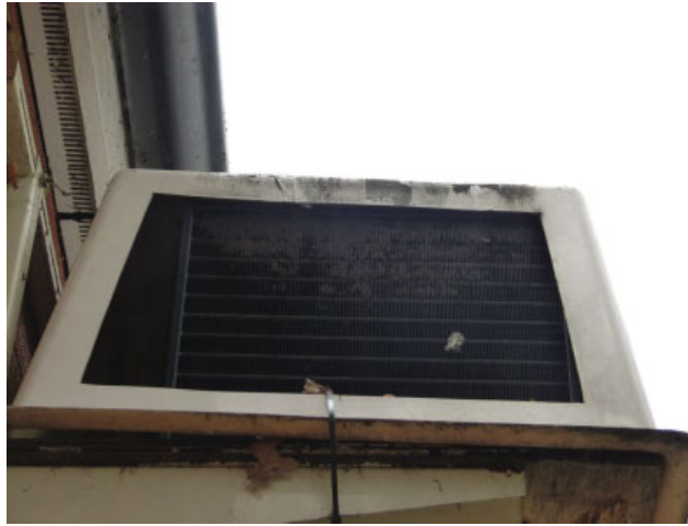
Figure 12.3 External refrigeration condenser unit fins need cleaning
