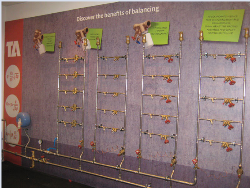
Figure 11.3 The importance of hydronic balancing can be practised on a purpose-built system
