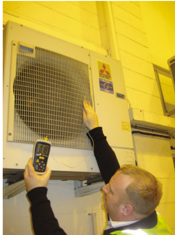
Figure 12.5 Measuring temperature performance and efficiency
