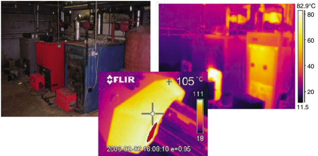
Figure T12.14 Boiler plant checks – insulation needed!
