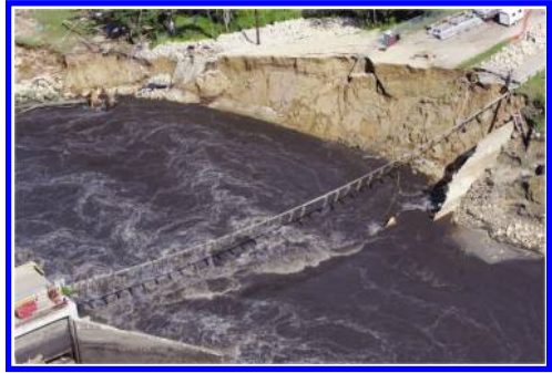
Figure 10. Breach gap with parts of the core wall.
