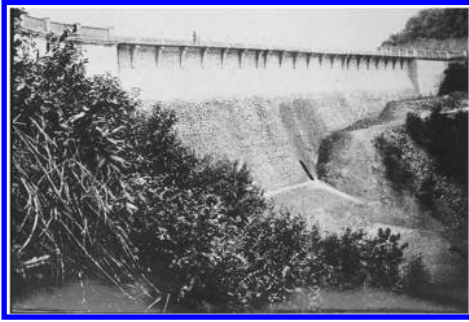
Figure 11. Sella Zerbino Dam before failure.
