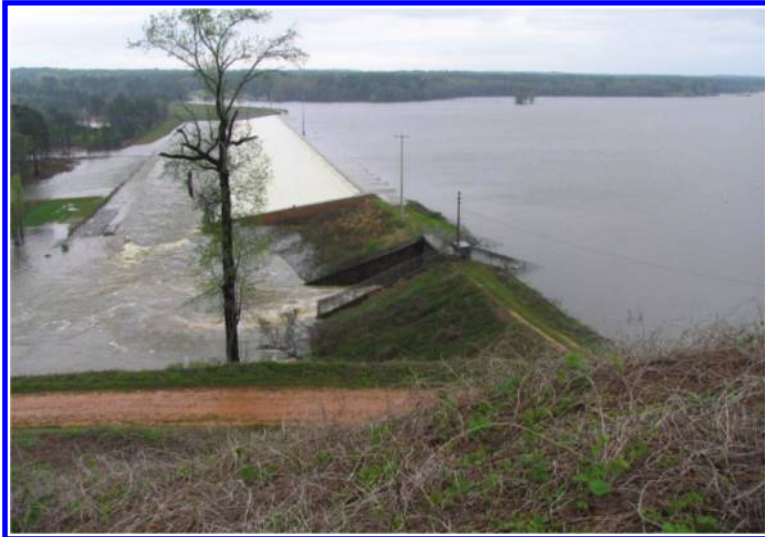
Figure 13. March 2005 overtopping event at Tholocco Lake Dam (provided by U.S. Army).
