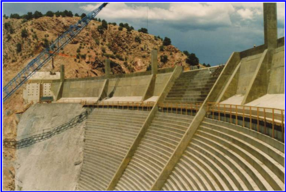
Figure 5. Concrete overtopping protection for Santa Cruz Dam in New Mexico. Splitter piers were provided for overtopping of the entire dam crest (Reclamation).
