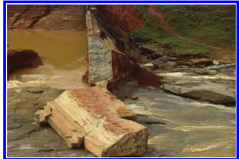
Figure 18. Detail of breach formation.
