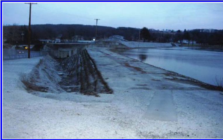
Figure 11. Lower Lake Royer Dam after 10 years of service.
