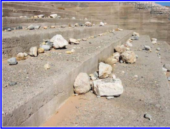
Figure 18. Boulders deposited on the RCC steps during 2005 storm. Photo taken in February 2006. Note limited wear of RCC steps.
