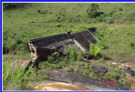
Figure 17. Poquim Dam after failure.
