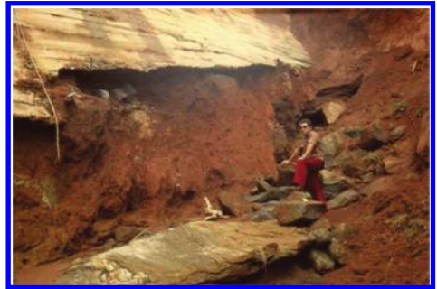
Figure 16. Erosion damage at the left abutment of Poquim Dam after the flood event in February 1979.
