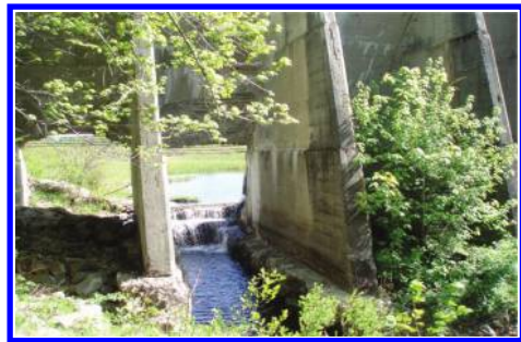
Figure 24. Breached Lake Leigh Dam.
