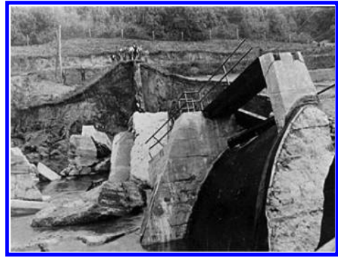
Figure 4. Fergus Falls Dam after failure.
