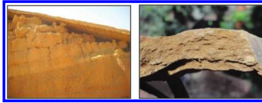
Figure 2. Left: Koumbri dam – stratification and thick compacted layers. Right: Guitti dam – foliation of the embankment is due to overcompaction insufficiently moistened fine materials.
