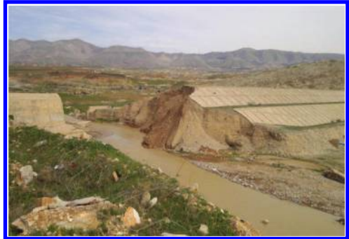
Figure 16. Chaq Chaq Dam after failure.
