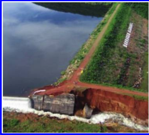
Figure 17. Algodoes Dam just before failure.
