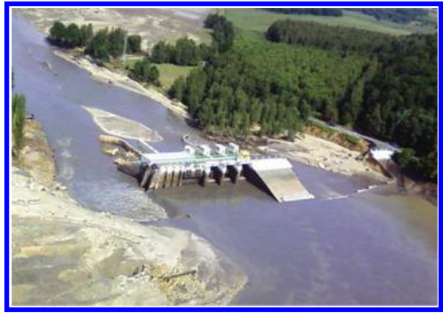
Figure 5. View of the completely eroded left wing.
