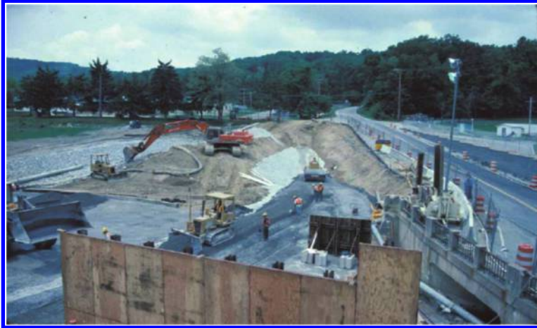
Figure 10. RCC construction at Lower Lake Royer Dam (provided by Maryland Department of the Environment).
