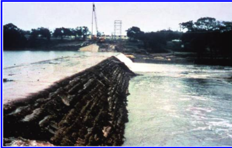
Figure 9. Kerrville Dam after major overtopping events.
