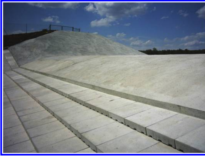
Figure 7. Detailed view of the upstream joint between the chute and the spillway inlet.
