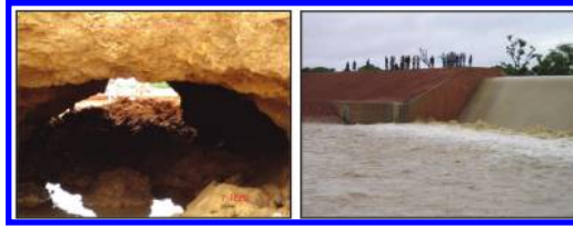
Figure 1. Left: Bampéla dam a hole in the embankment. Right: Gazandouré dam-spillway and leak at the contact with the embankment on right side.
