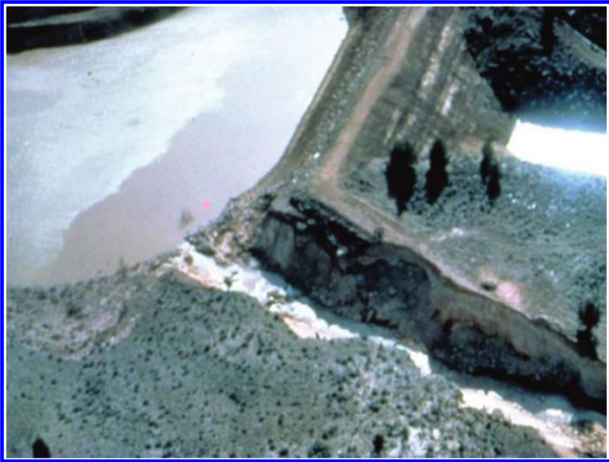
Figure 1. Unlined spillway erosion ( http://www.damsafety.org/ ).
