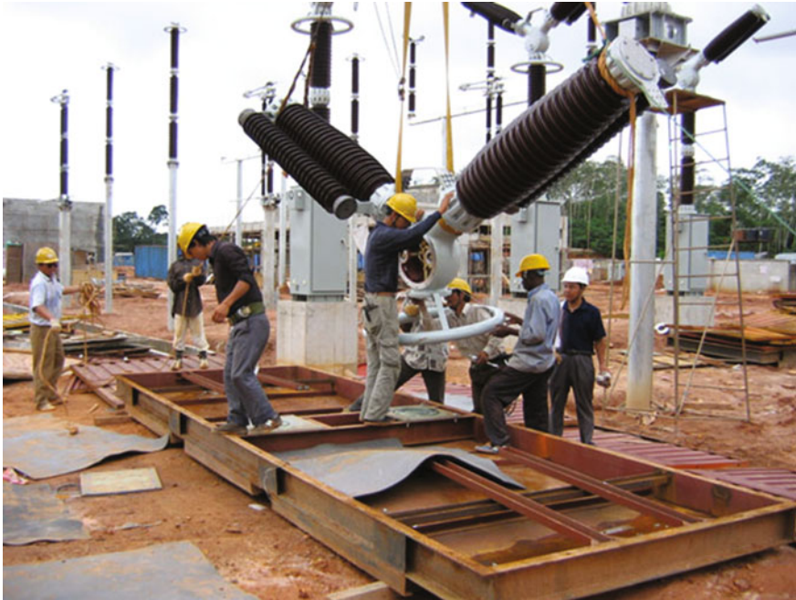
Fig. 8.12 Case Study 4 project site (during an earlier stage of Phase 2 of the project)
