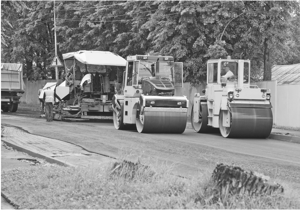
FIGURE 10-4 Many steps and considerations are taken during the construction phase of a project, in which plans that were designed on paper are now taken on-site and implemented on the ground. Image acquired from depositphotos.com.
