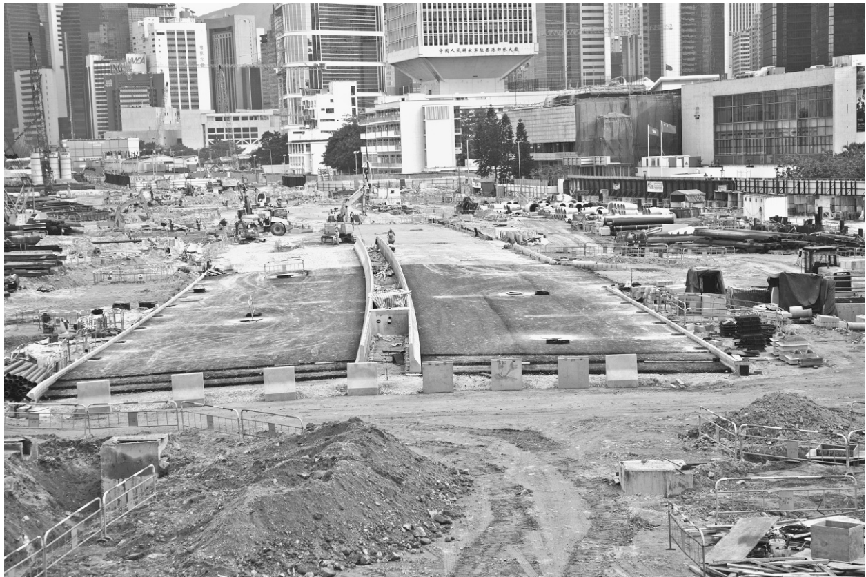
FIGURE 10-6 Road construction near the harbor of Victoria in Hong Kong. Image acquired from depositphotos.com.
