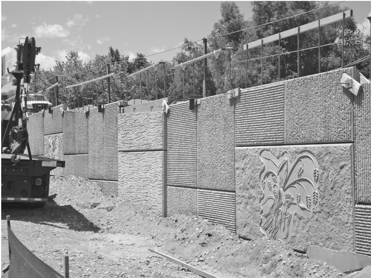
FIGURE 10-5 Mechanically stabilized earth panels, featuring concrete textures, are pieced together to form a retaining wall. This construction process helps minimize construction impacts because the panels can be premanufactured and shipped to the site. Image courtesy of Colorado Department of Transportation.
