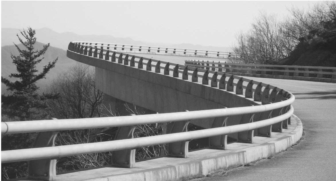
FIGURE 8-32 The Linn Cove Viaduct snakes around the slopes of Grandfather Mountain along the Blue Ridge Parkway. Image courtesy of Wikipedia Commons.
