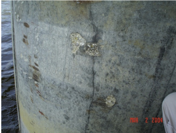
Figure 3.4 Longitudinal crack in prestressed concrete cylinder pile.
