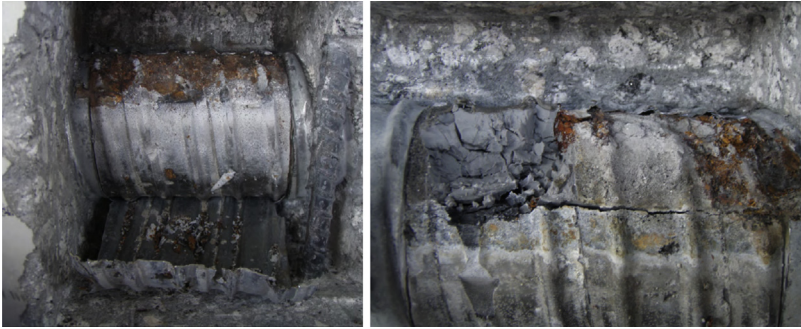
Figure 3.7 Corrosion of metal duct with deficient grout. Photos courtesy of Florida Department of Transportation.
