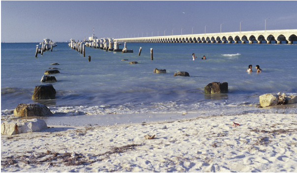
Figure 4.2 The pier on the right was built with stainless-steel rebar in Progreso, Mexico between 1938 and 1941. The remains of a parallel pier built 30 years later with black steel rebar can be seen in the foreground.
