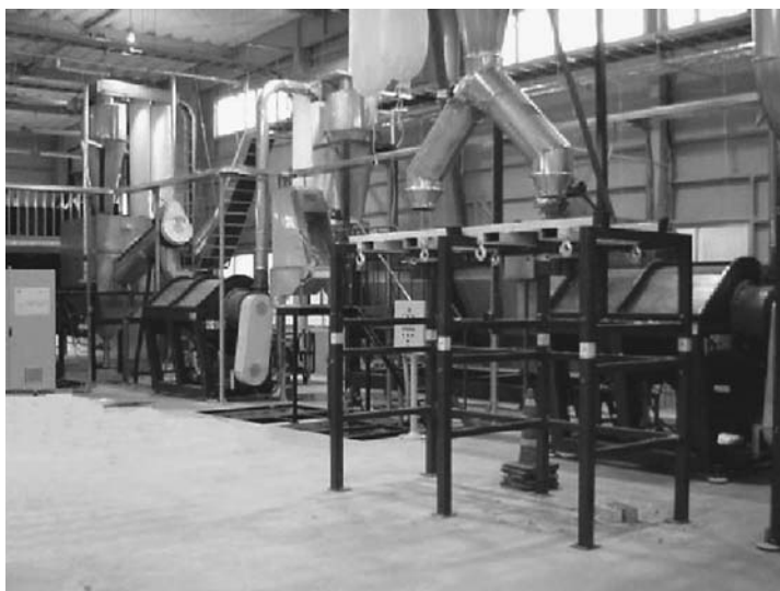
FIGURE 18.19 LDPE film recycling plant.
