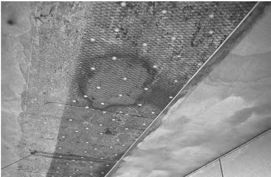
8.4 Three stages of application of a titanium mesh to the underside of a concrete slab with corrosion due to penetrated chloride; left part of photo : prepared surface; middle : titanium mesh attached (note big repair patch and plastic fixing pins); right : shotcrete overlay applied.
