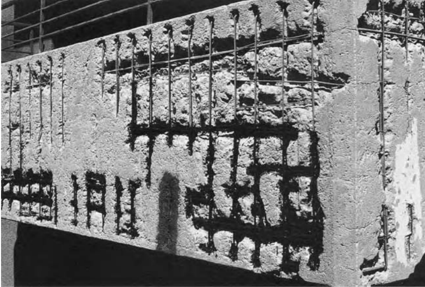
6.5 Reinforcing exposed by blasting.
