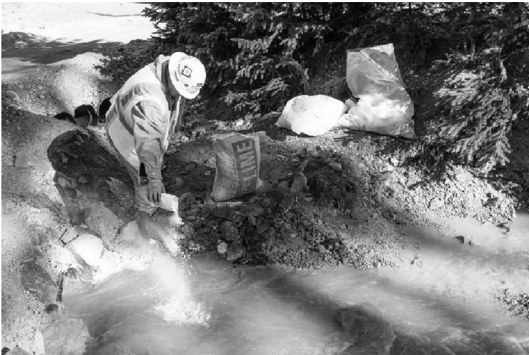
FIGURE 8.4 As water exits the mine, it flows into a system of four treatment ponds. The treatment ponds provide retention time to allow the pH to adjust. Here, lime is added to a settling pond to assist in the pH adjustment of the water prior to discharge to Cement Creek and the Animas River on August 14, 2015. (From USEPA, Emergency Response to August 2015 Release from Gold King Mine , U.S. Environmental Protection Agency, Washington, DC, 2016, http://epa.gov/goldkingmine . Photograph by Eric Vance/EPA.)
