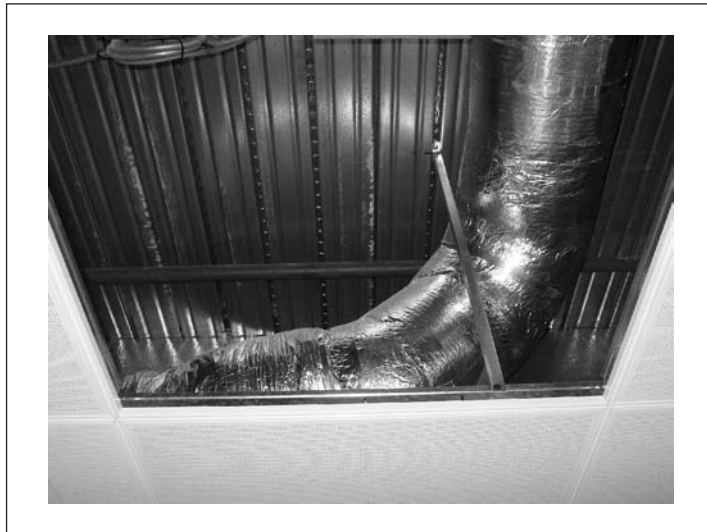
Figure 13.10 ● Ducted services for ventilation/air conditioning housed within the ceiling void. Access is easy using the jointed ceiling.
