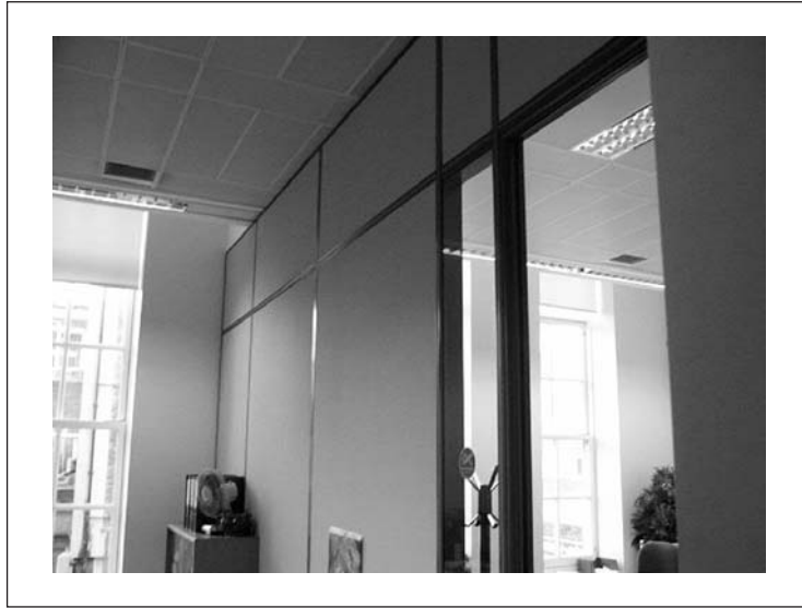
Figure 13.21 ● A typical demountable partition.
