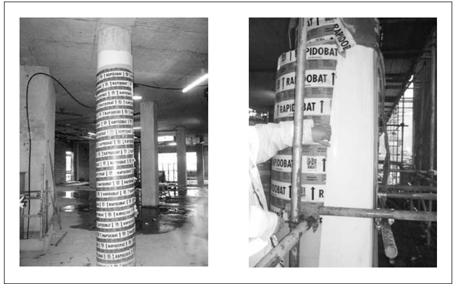
Figure 7.4 ● These photographs show round section columns being cast in situ with the aid of single use cardboard formwork. The cardboard tube is lined with smooth PVC to create a finish of high quality. Figure 7.5 indicates the components of this system.
