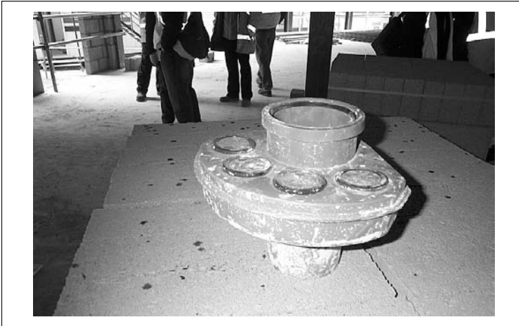
Figure 3.7 ● An 'elephant's foot' waste pipe manifold.
