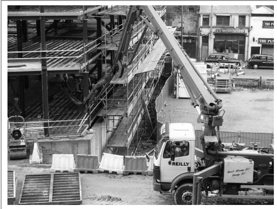
Figure 7.3 ● A concrete pump being used to facilitate the casting of concrete floors to a steel framed building.
