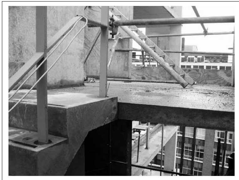
Figure 11.16 ● Precast stairs being used for a multi-storey building. Here we see the stair at the junction with the landing. Note the difference in surface level due to the need to accommodate a screed finish to the landing.
