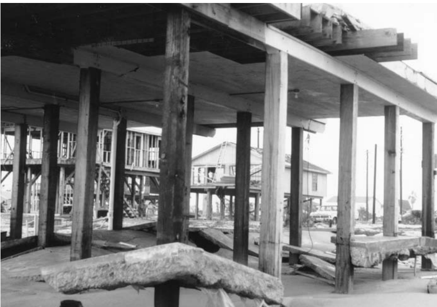
FIGURE 12-9 Remains of oceanfront home elevated on pilings embedded in concrete after Hurricane Alicia in 1982 at Galveston Island. (Photo by author.)
