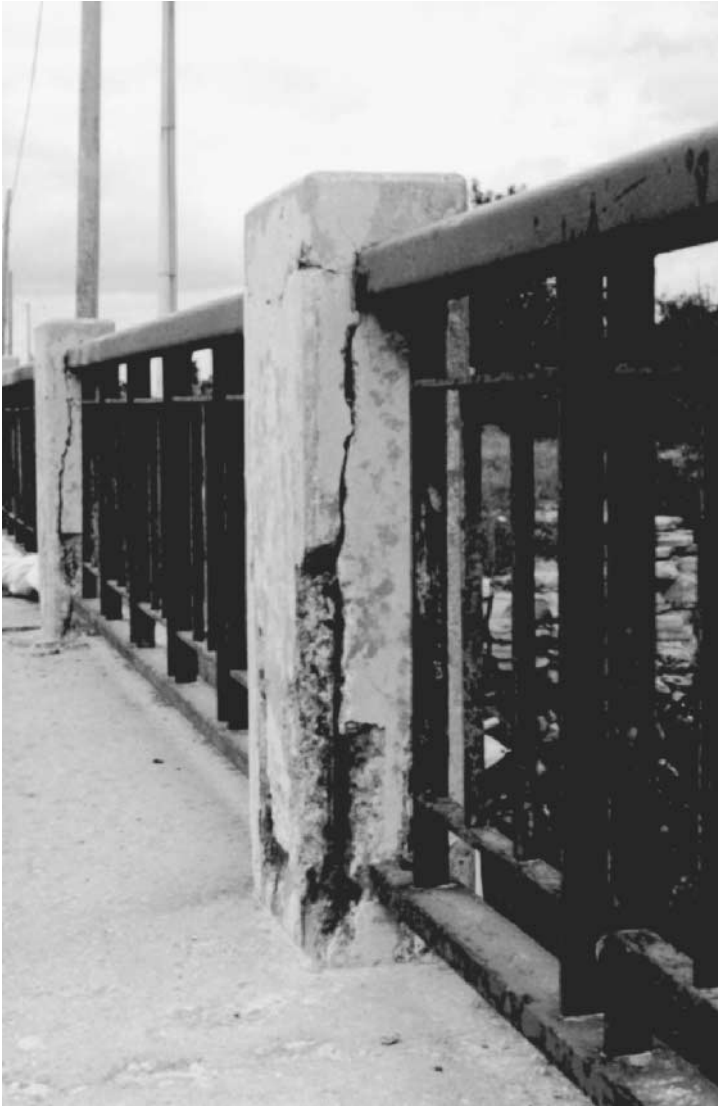
Figure 2.28 Concrete degradation caused by rebar corrosion damage near Kingston, Ontario. This bridge underwent extensive rehabilitation shortly after this picture was taken.
