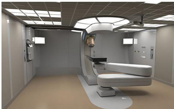
Fig. 39.2 The Still River PT system treatment room
