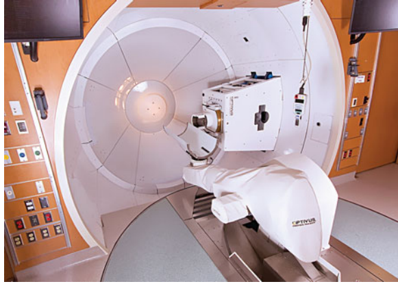
Fig. 34.5 Robotic positioner in place, Gantry Room 1, James M. Slater, M.D., Proton Treatment and Research Center
