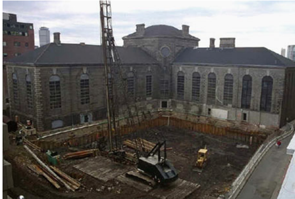
Fig. 35.4 Start of construction of the Proton Therapy Center in 1995 in the narrow space of the MGH parking lot, formerly the exercise yard of the Charles Street Jail
