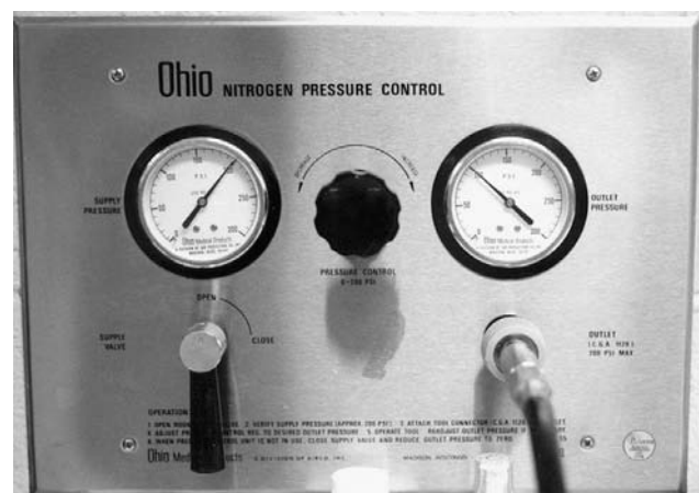
Figure 4.3-2 OR wall outlet for nitrogen gas.
