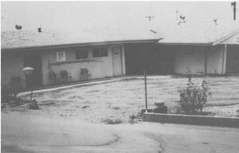
FIGURE 13–5. A motel built on a landfill that experienced differential settling
